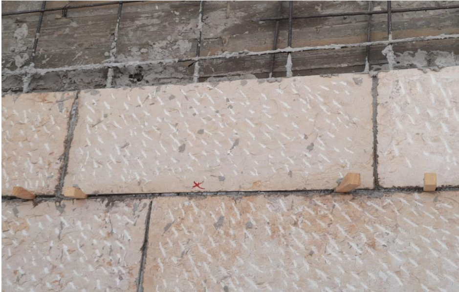
Pointing on the defected stone to be removed
