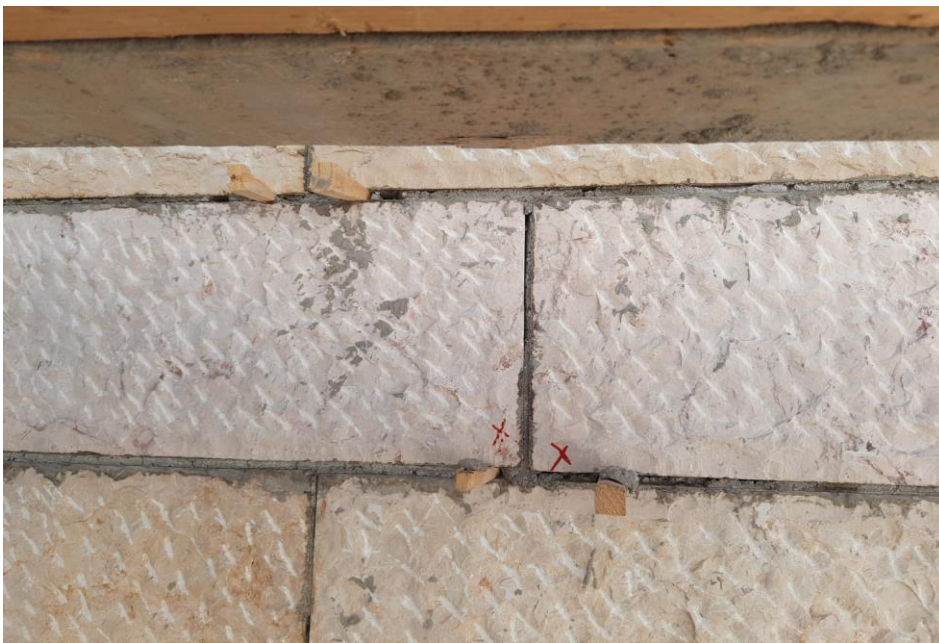
Pointing on the defected stone to be removed
