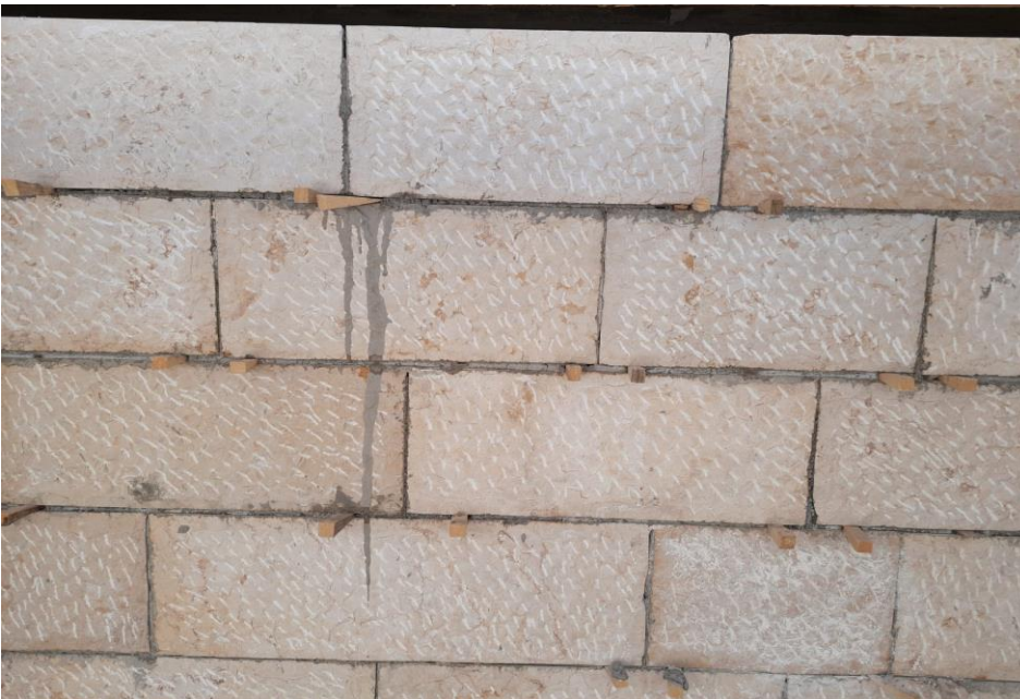
Remarks on the stone work as per the report
