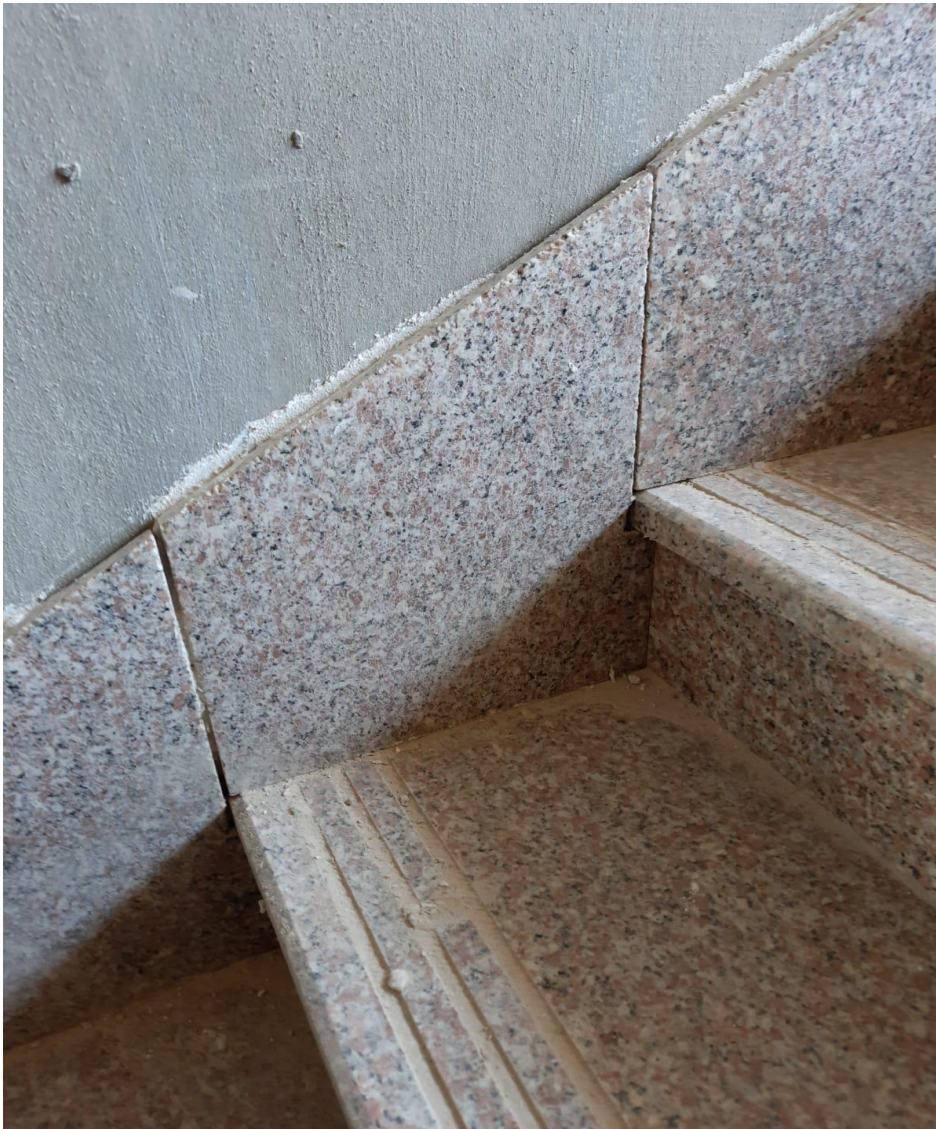
Defected granite tiling
