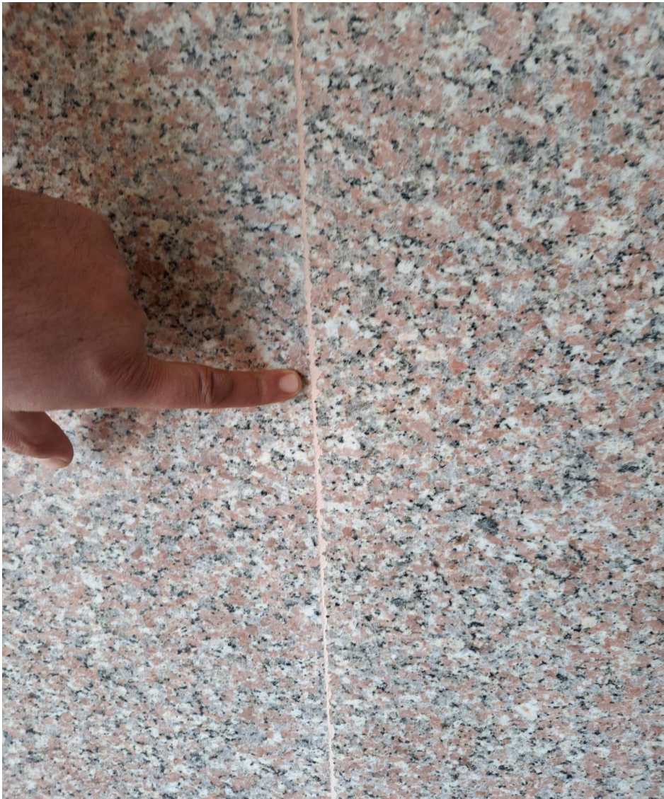
Defected granite tiling
