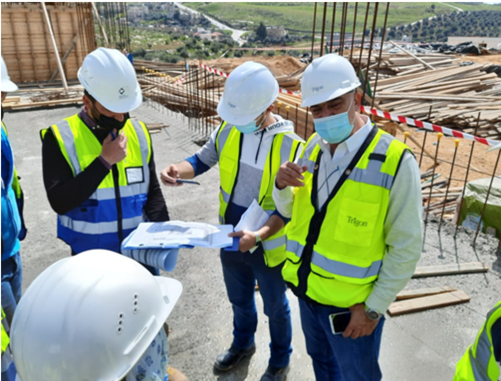
Discussing the work and boundary walls progress and relocation of the Engineers offices before starting executing external yard
