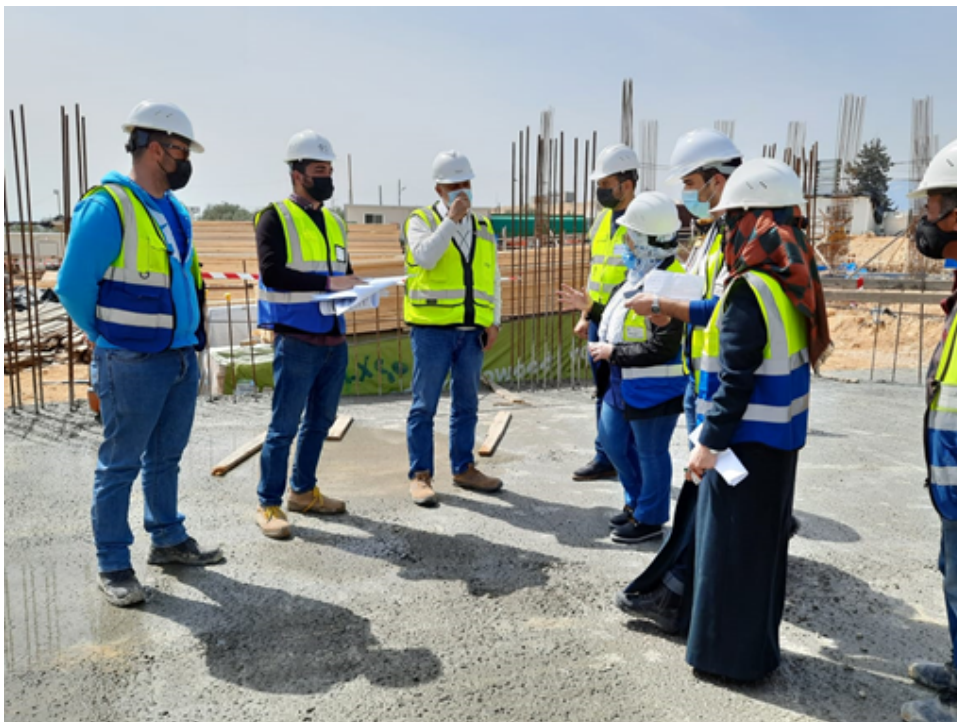
Discussing water tank location as provided by the Designer, and the issue of the plot limit which is still pending
