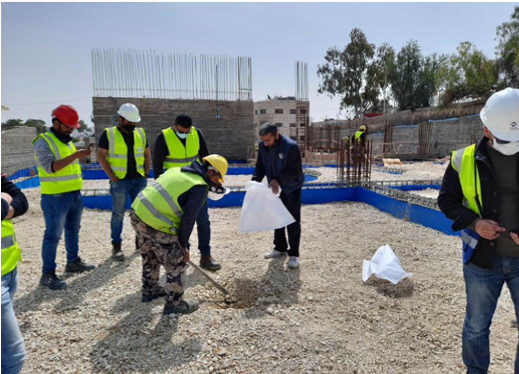
Taking Base course samples by laboratories and quality control department in MPWH- (14/03/2021)
