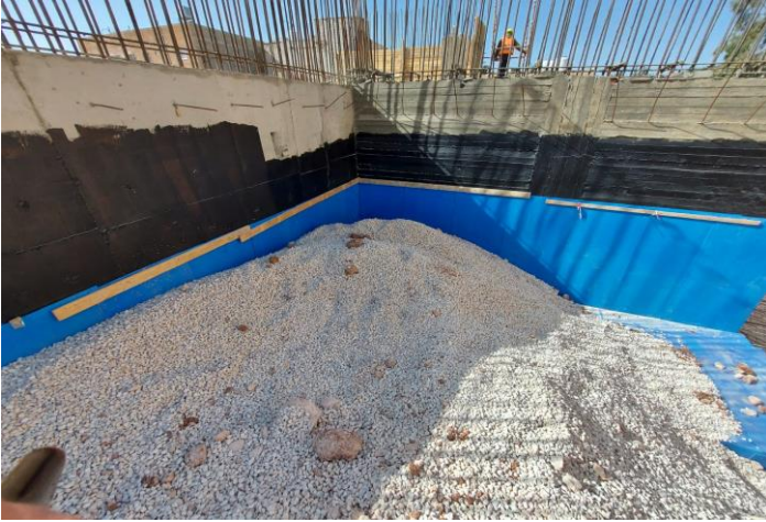
Conducting back-filling work without doing the appropriate insulation work
