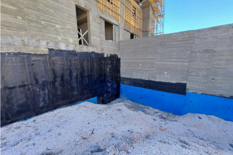
Remedy work has been finished (removing back-filling and applying waterproofing membrane as per specification)
