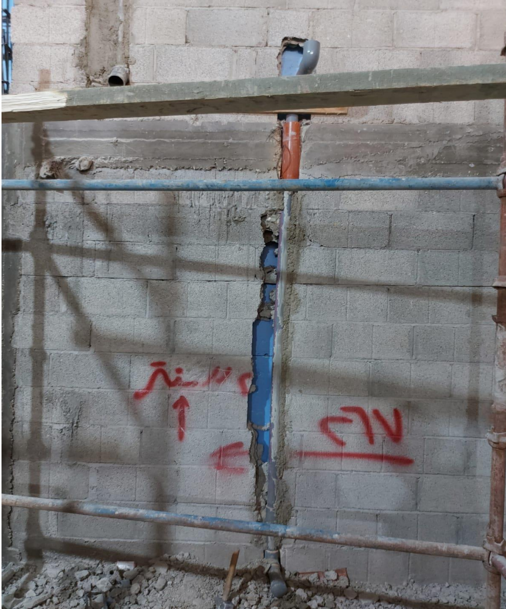
Example of defected work
