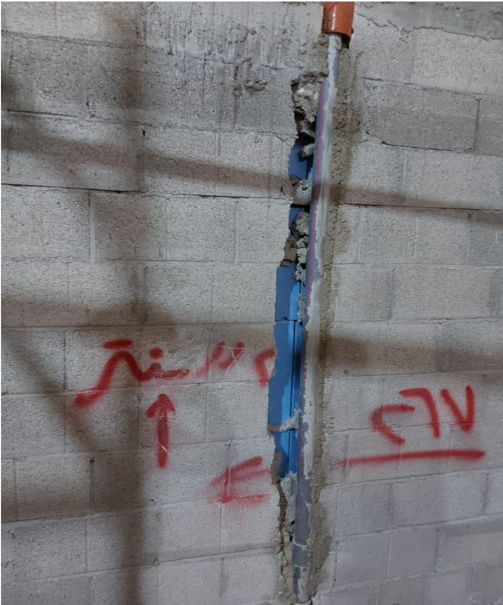
Example of defected work
