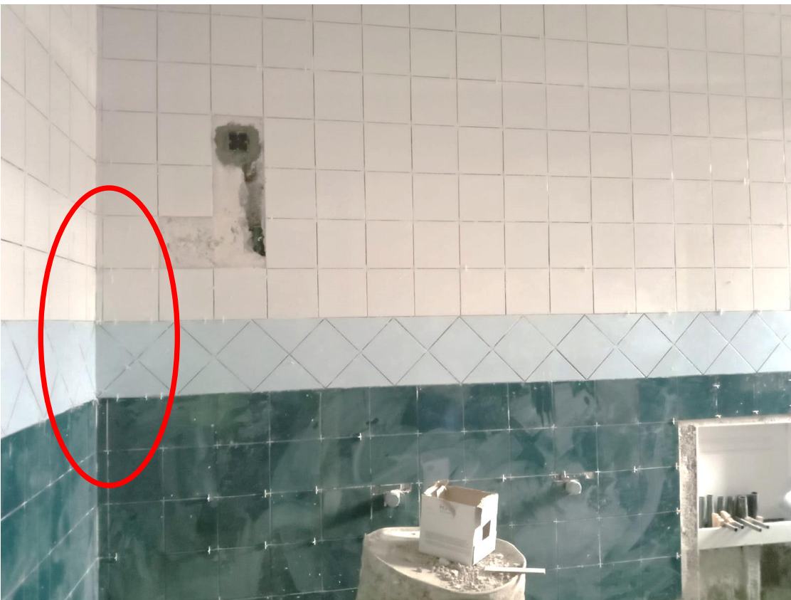
The supervision team observed that the tiling work at one wall does not comply with the shop drawings due to defect in the starting points of tiling
