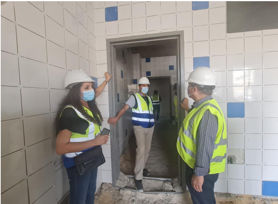
The supervisory team conducted a general check on the installed door frames and their relation with the wall tiles with reference to the design drawings
