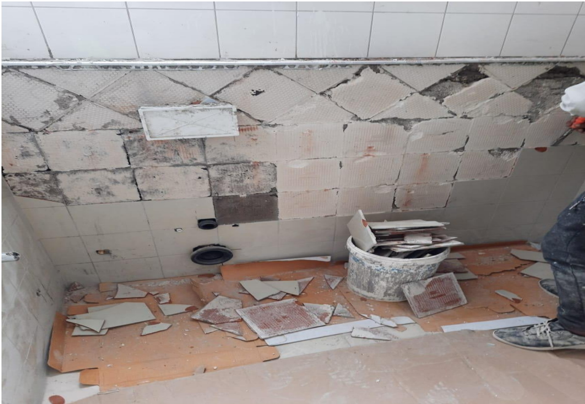
Removing of wall tiles due to the failure of adhesive material
