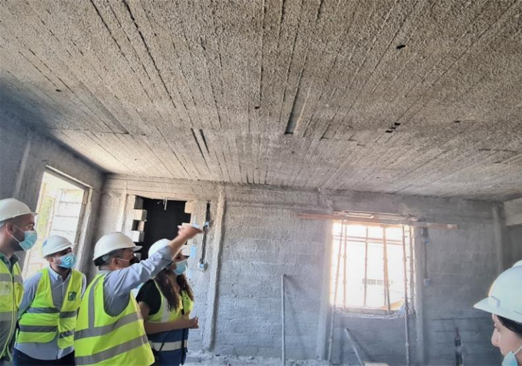
Irregularity in the formwork of the slab
