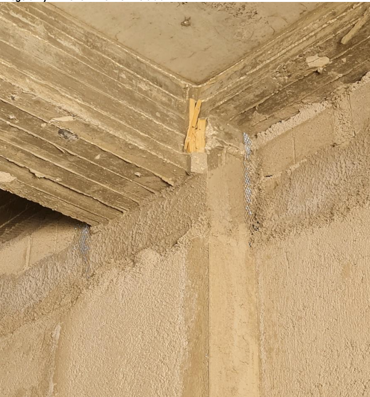
Remaining wooden pieces in the slab
