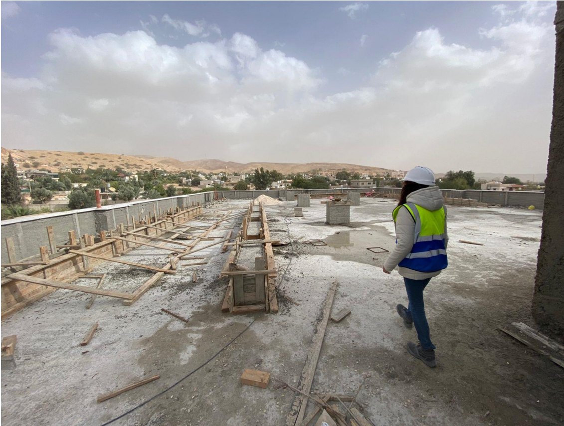
The concrete bases of the mechanical equipment at the roof are under construction
