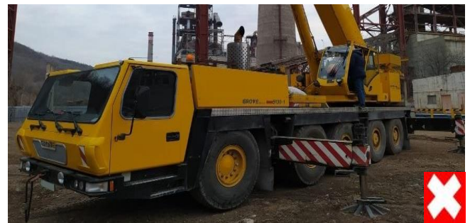
Figure (2): The Ground is Not Stable
