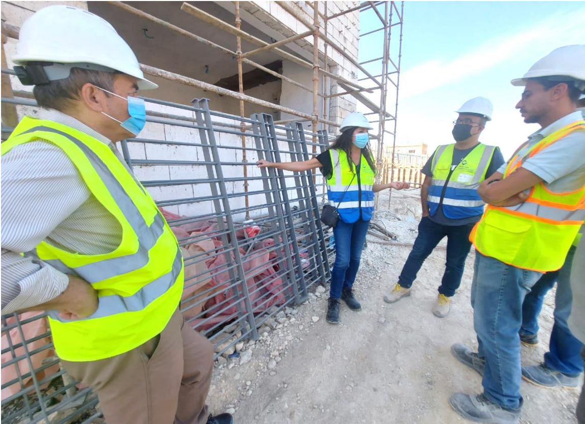
The Contractor imported the steel grill protection and the supervision team inspected before installation
