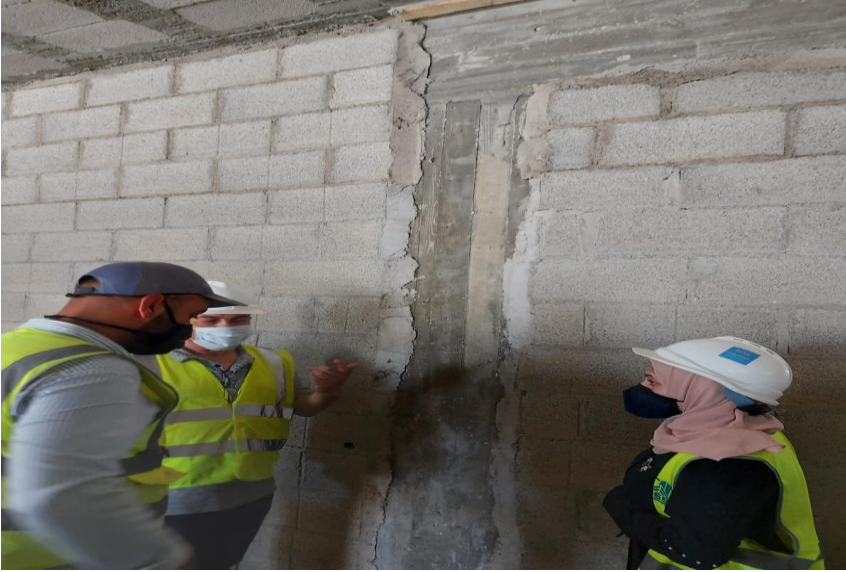
The blockwork is not in line with columns
