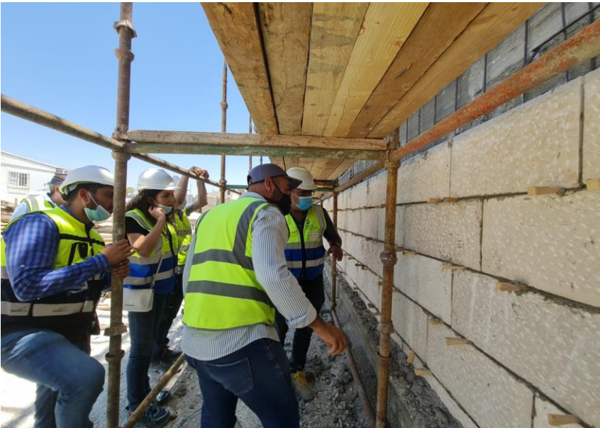
Remarks on the stone, broken edges, gaps not unified, chiseling pattern not unified, ...
