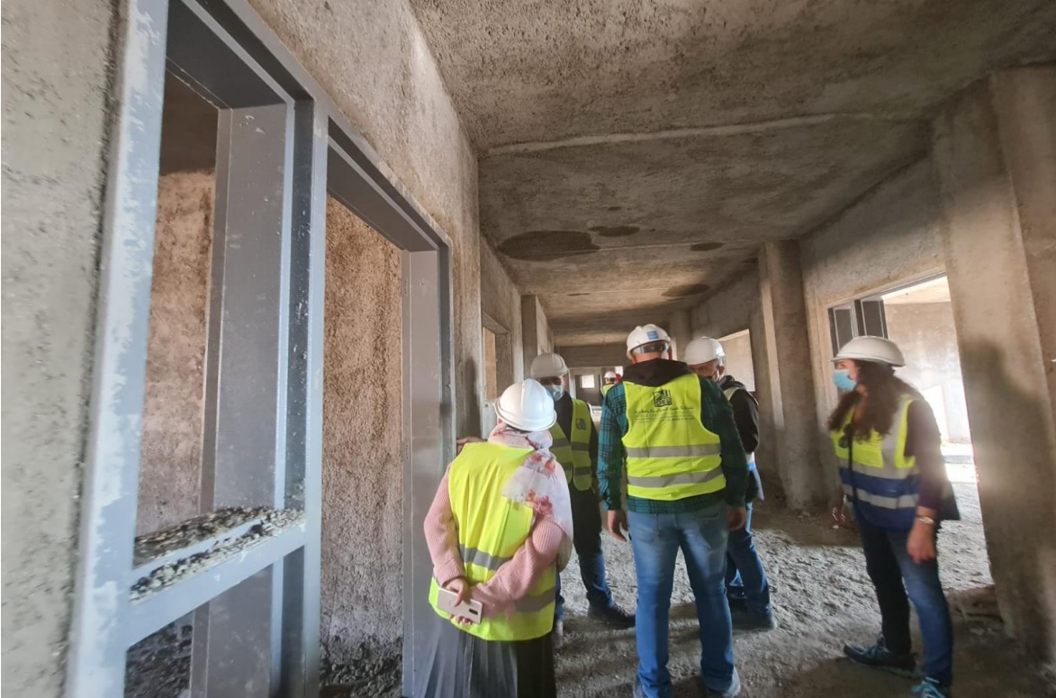
Dirt and cement mortar residues on door frames
