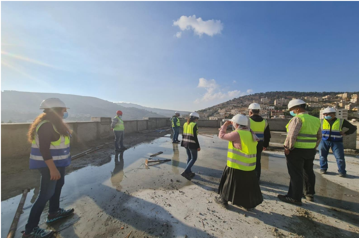
Rain water gathering at the roof
