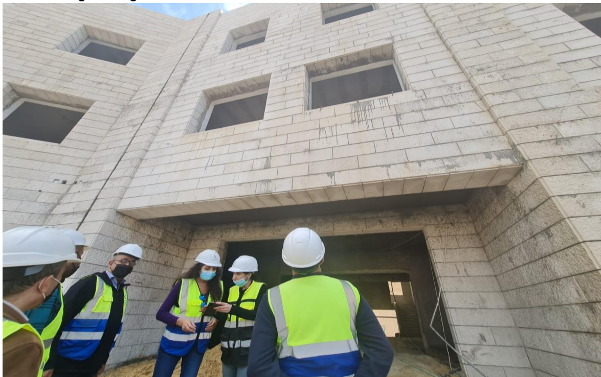
Penetration of rain water through the walls
