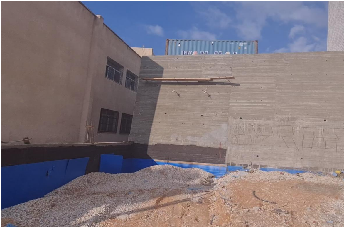
Cartonal sheets protecting the insulation of boundary walls not completed
