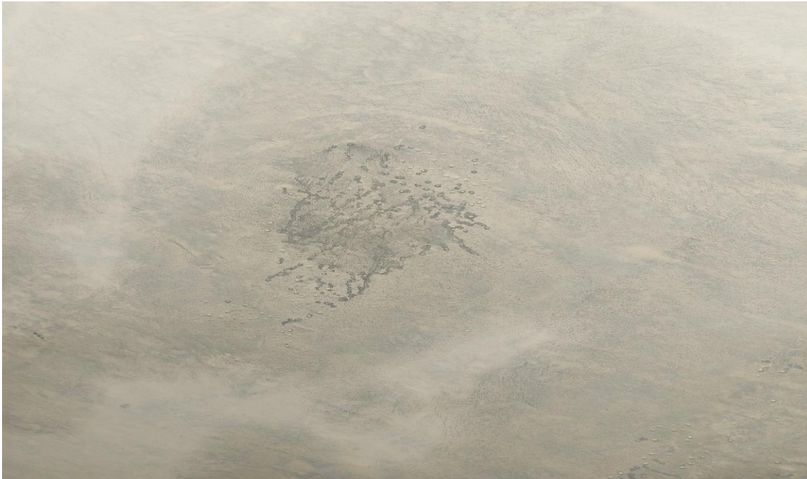
Penetration of water at the ceilings
