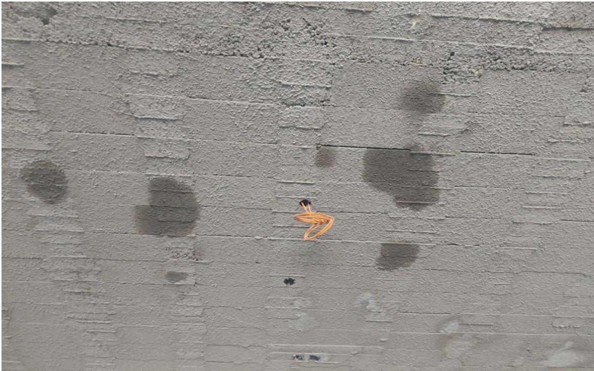
Penetration of water at the ceilings
