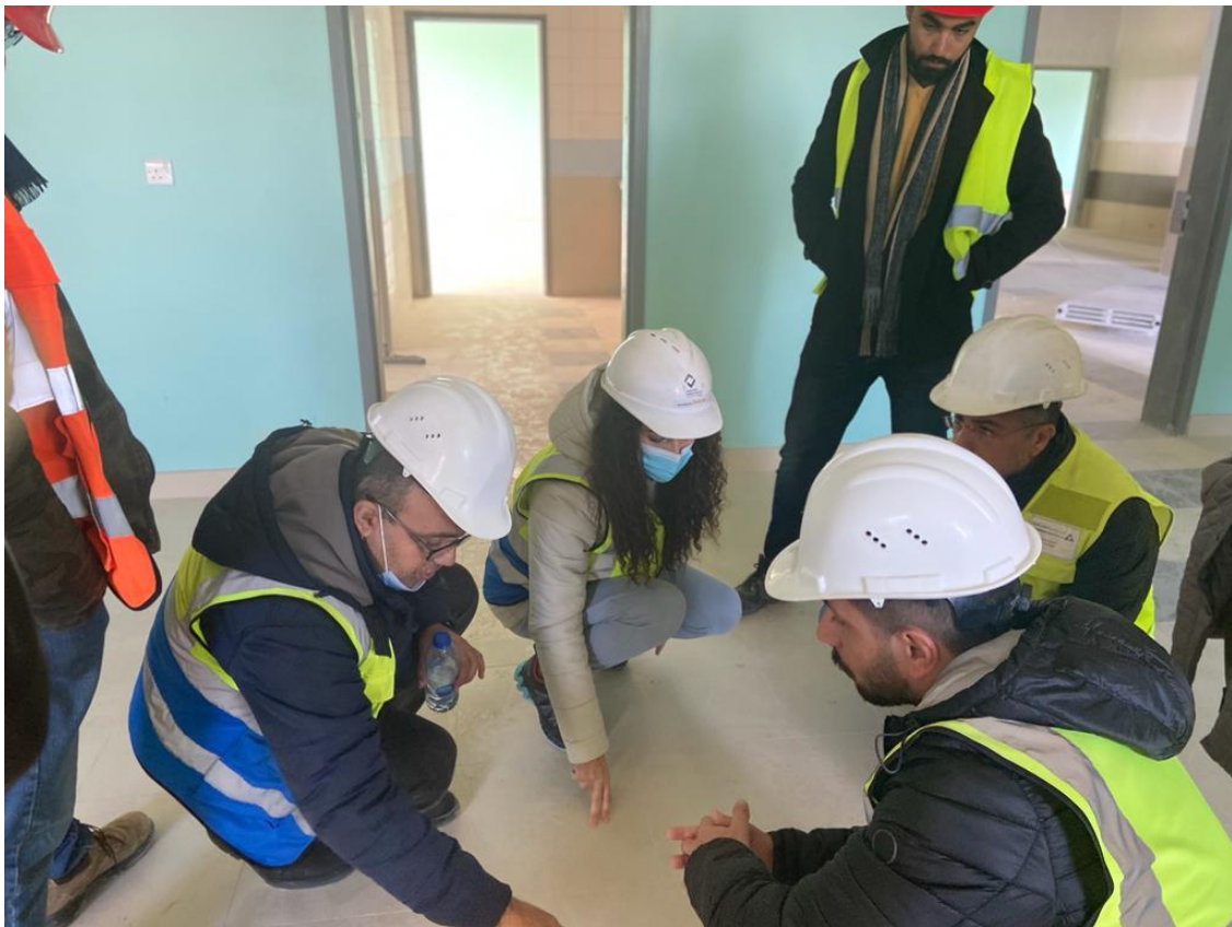
The supervision team inspected the floor tiles at the mock-up room after the Contractor conducted rectification work by replacing number of defected tiles. The team observed that the defects (teething and uneven face) in general still remain
