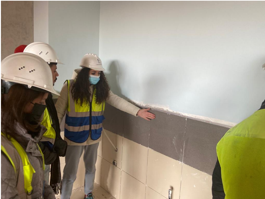
The team inspected all the installed beads at the ends of tiled walls
