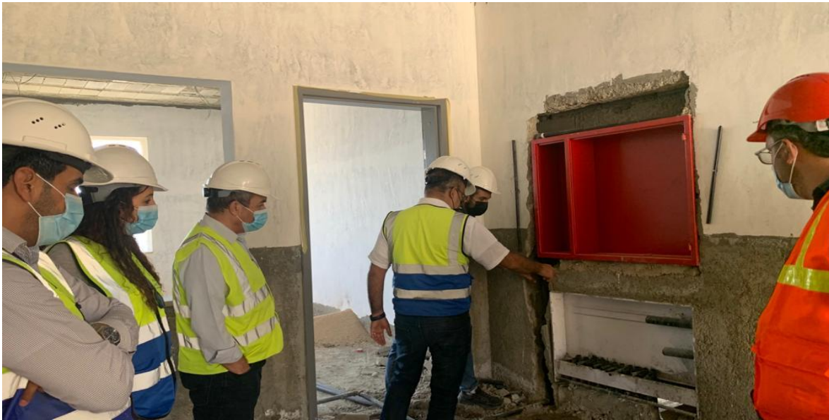
Defects around fire hose cabinet and mechanical cabinet
