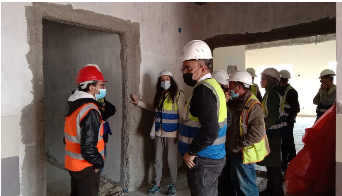
The frames of fire rated doors still have not been delivered to the site
