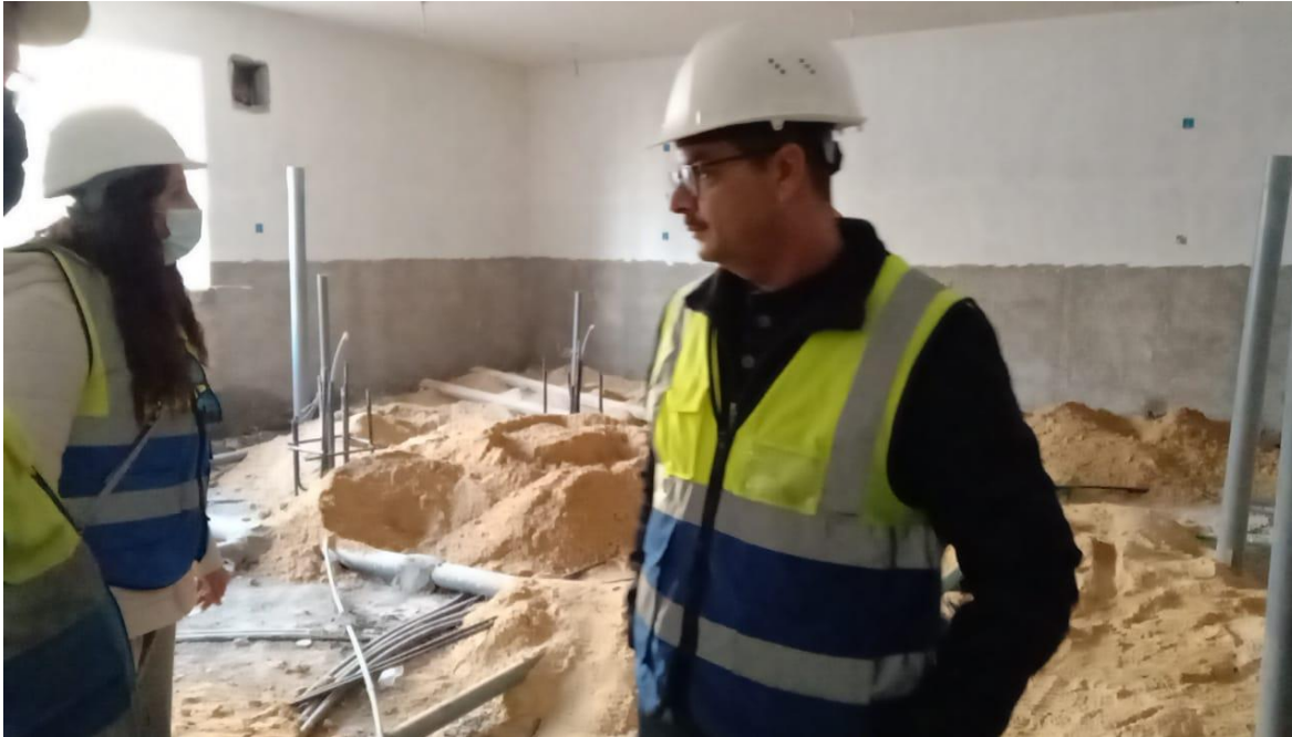
The ongoing electro-mechanical works have been inspected in the presence of our electrical engineer
