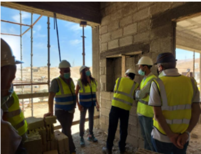
One location of "Fire Hose Rail Cabinet" was checked and remarks were given to Contractor regarding the finishing of the double wall
