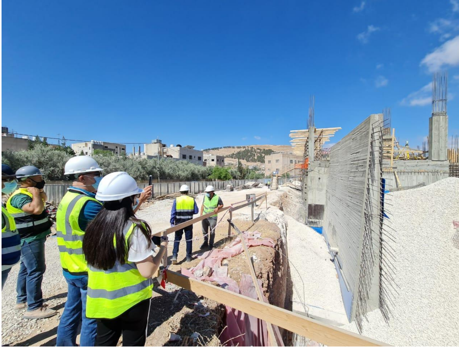
Checking safety measures beside excavation trench and the execution of insulation at vertical element
