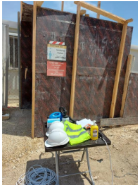
← Sterilization and signing visitors' attendance sheet at the entrance of the site, complying with Covid-19 Protocol ↙
