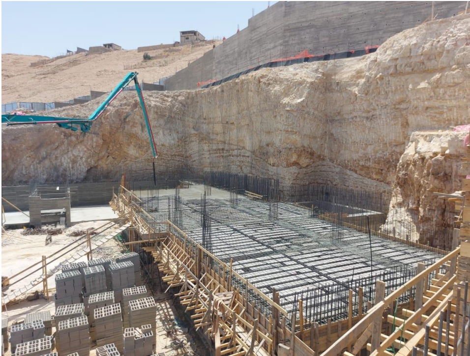
Concrete casting for slab for the first floor at zone B of school building
