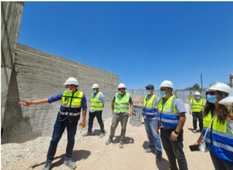
Inspecting casted vertical elements of Basement Floor and ground floor at zone B
