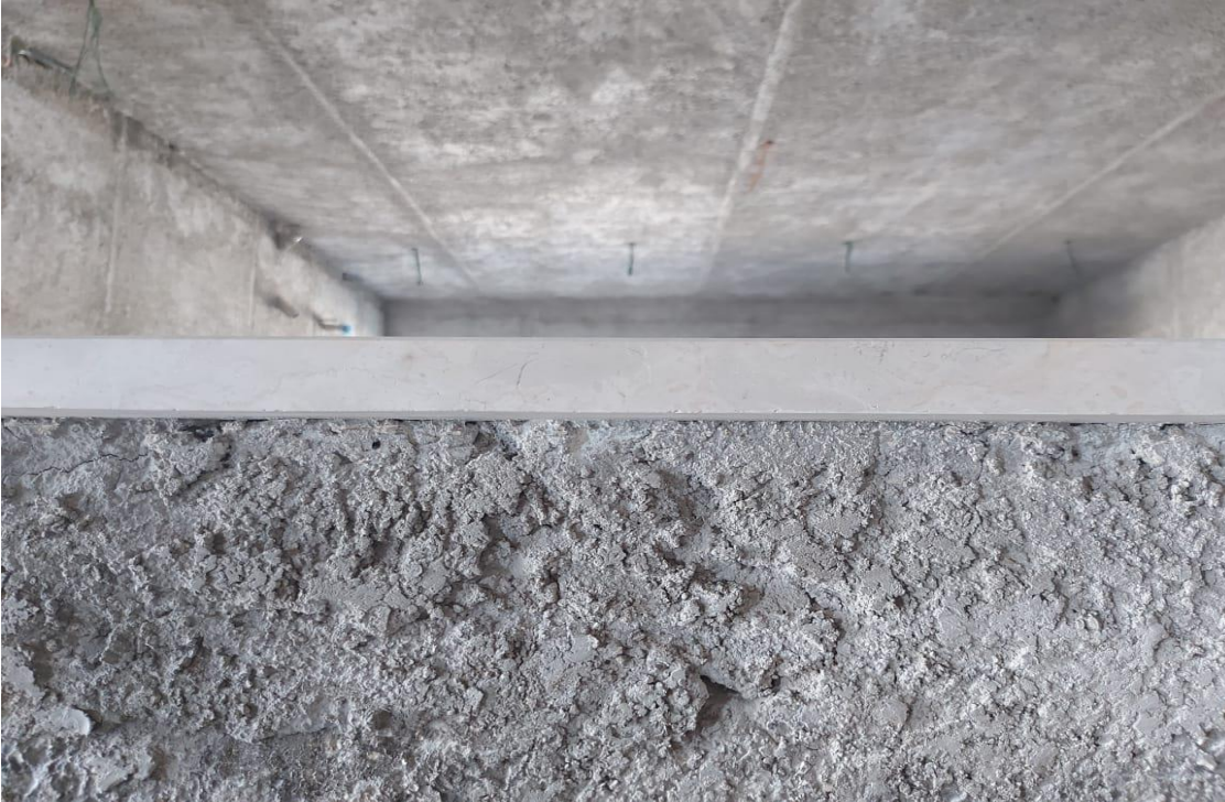
Defects in the sill and installation at lower level
