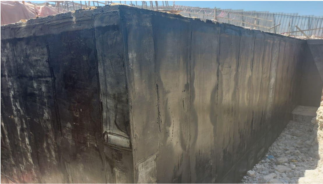
Unprotected waterproofing sheets for watertank and septic tank
