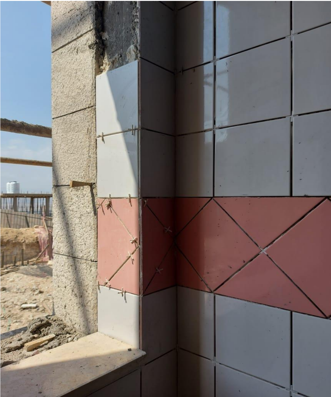
No tiles beads used in the tiling
