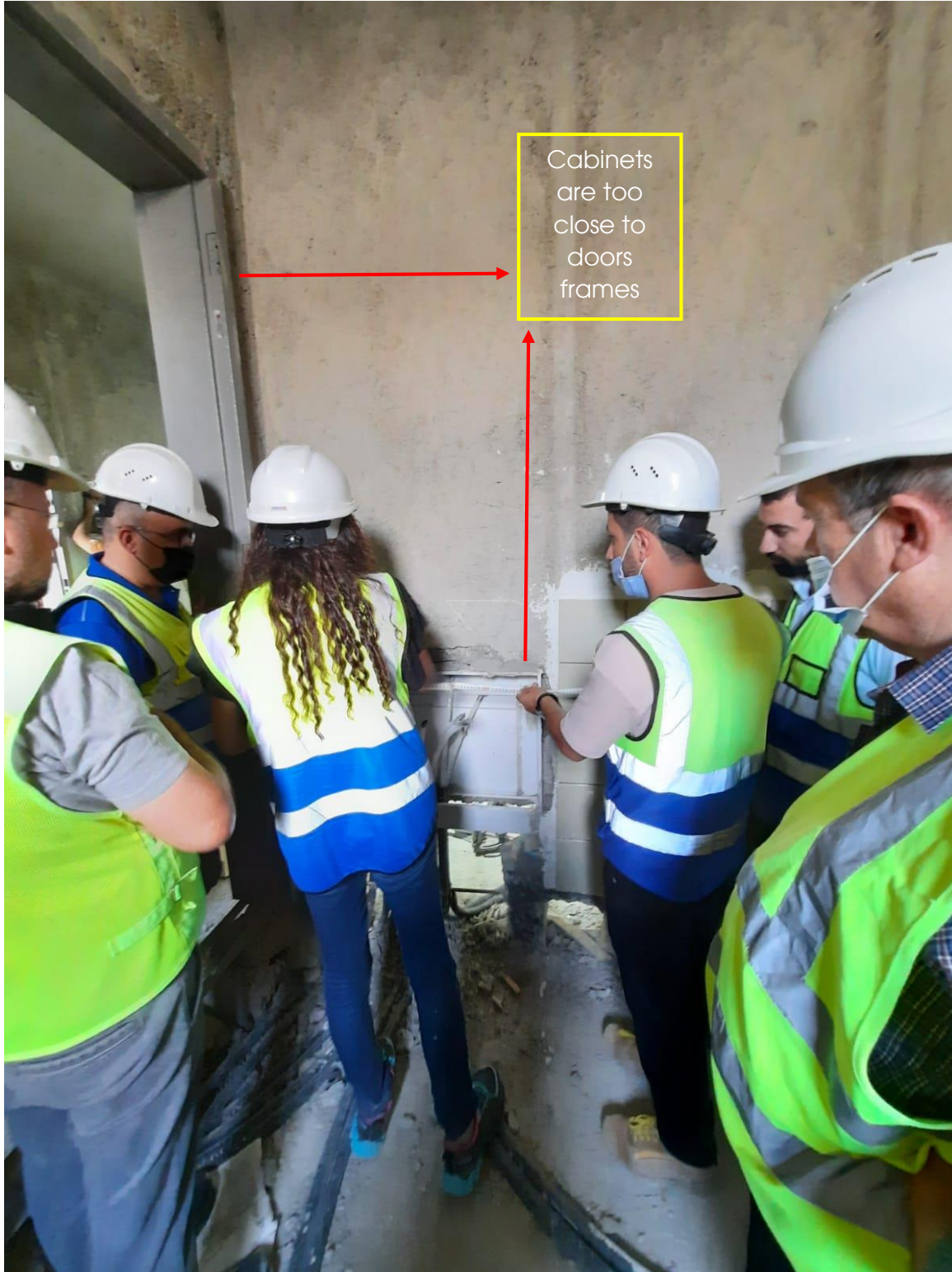
Mechanical cabinets in the toilets area and their location in relation to the door frames
