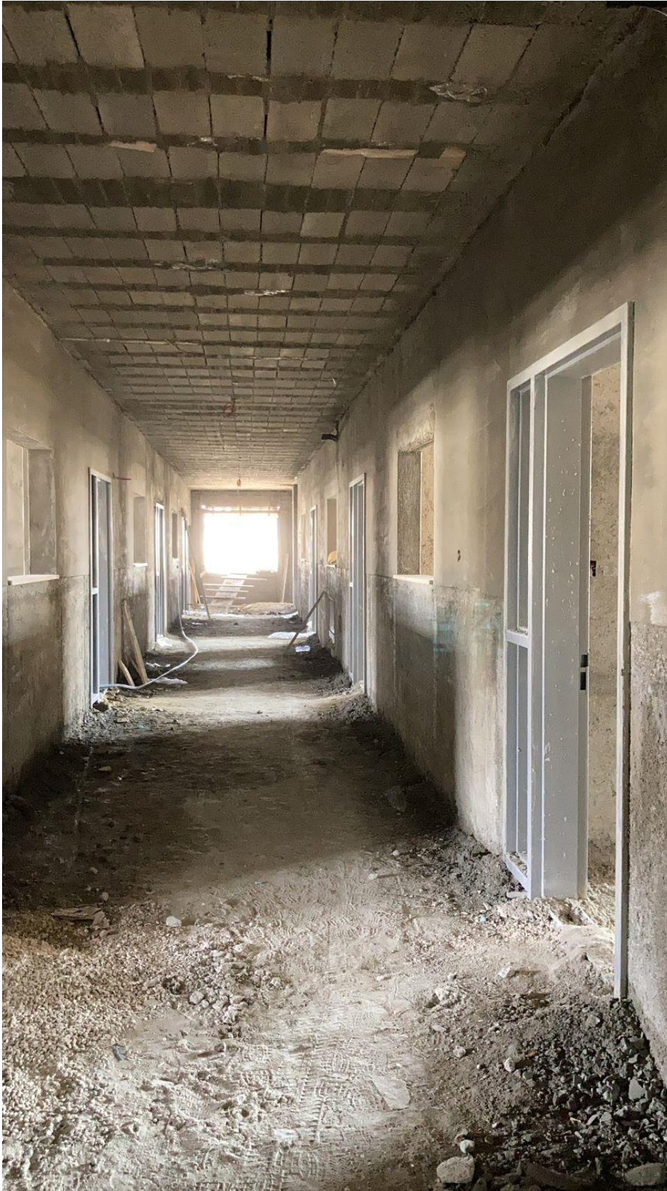
A view for the corridor showing the installation of door frames- Ground floor
