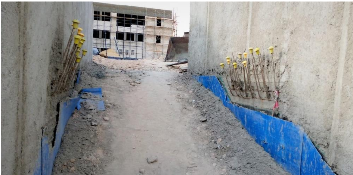
The visiting team observed applying caps at the ends of reinforcement bars and stressed on their importance to insure safety
