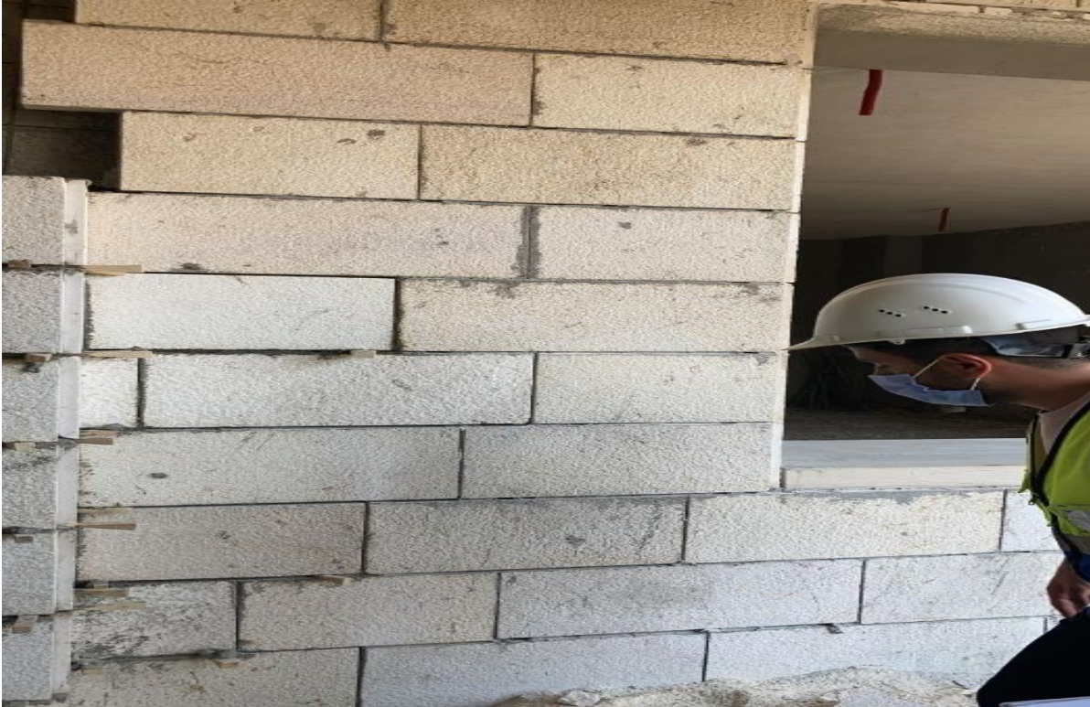
Defected stone building
