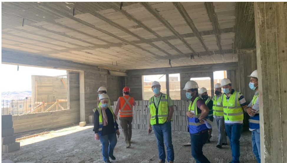
Different quality issues were discussed regarding the block works and the fixation of the Polystyrene boards
