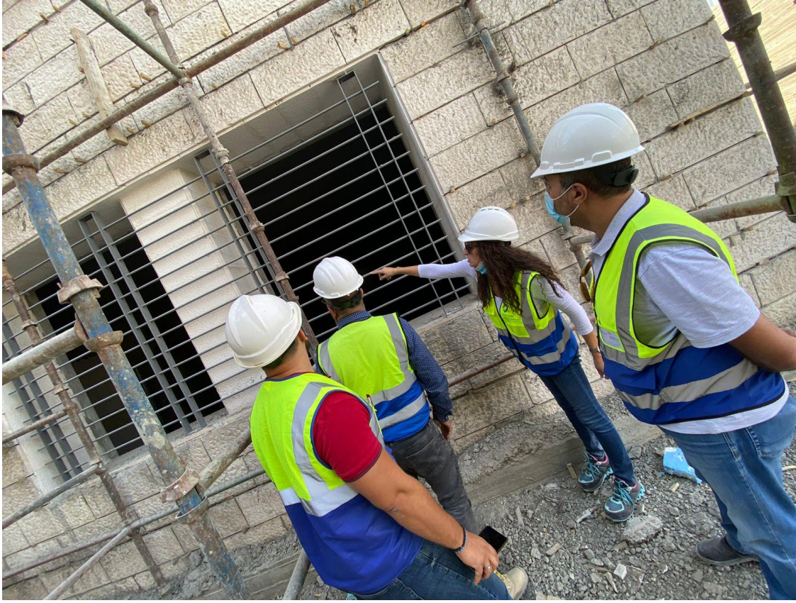
The installed sample of steel protection grill for window was inspected by the visiting team
