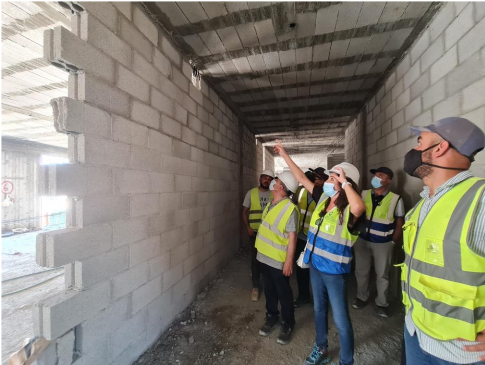
Voids within block walls were noticed and the Contractor was instructed to close them correctly
