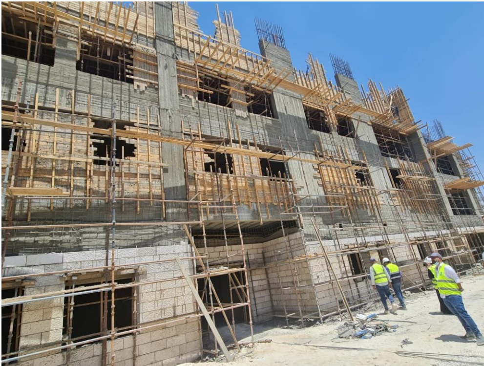
-The Contractor is carrying on shuttering works for concrete walls behind stone for ground and second floors -Starting stone works (Zone A)
