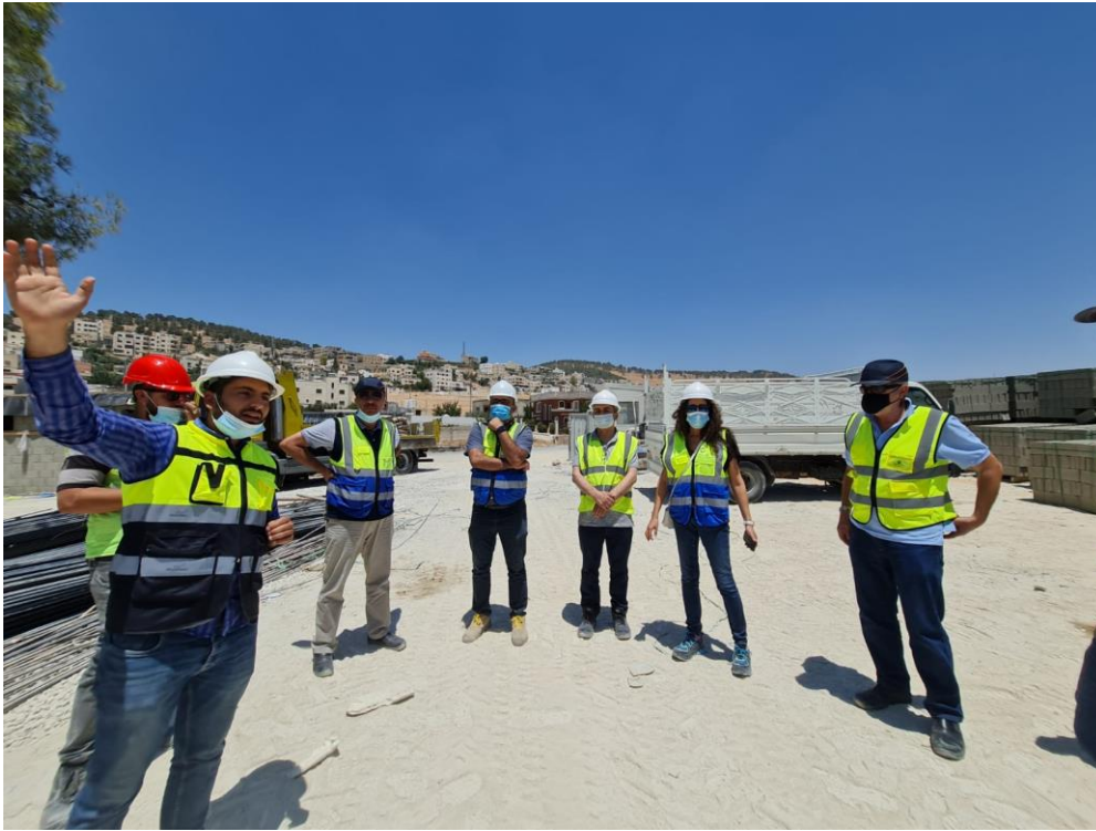
Sadam Boqain/ supervision site engineer gave a brief on the safe routes at the site
