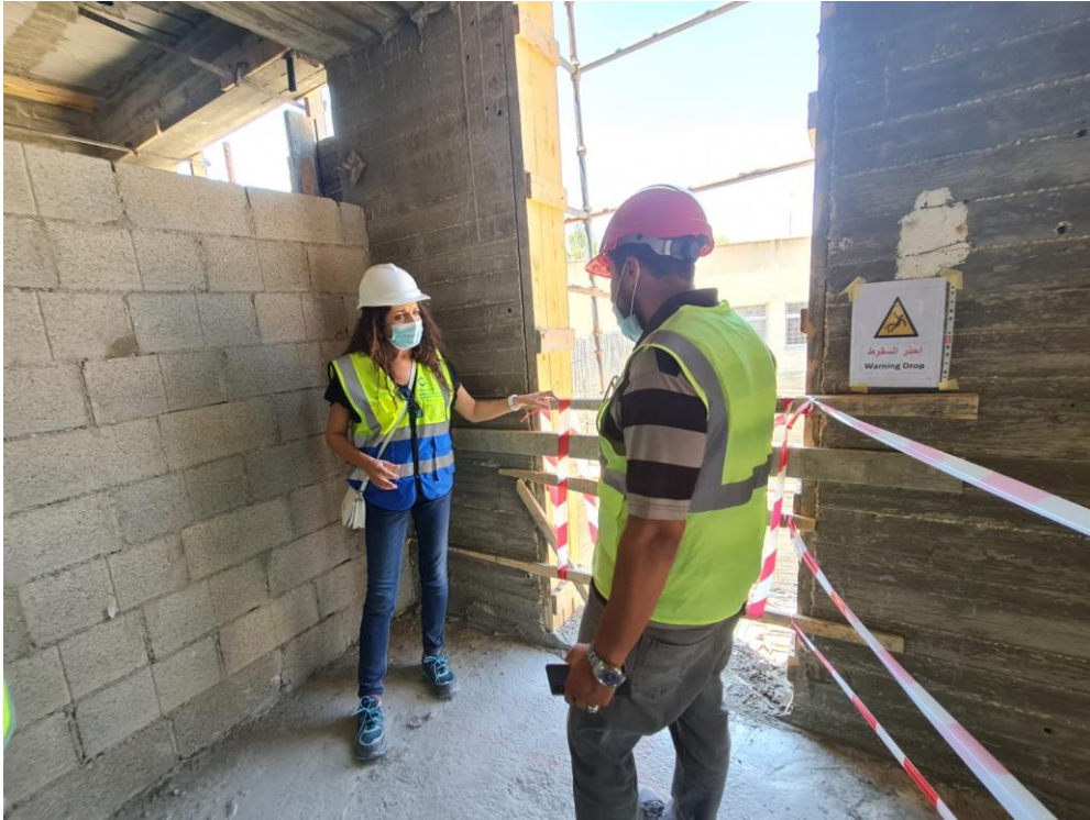
Acceptable safety protection for openings
