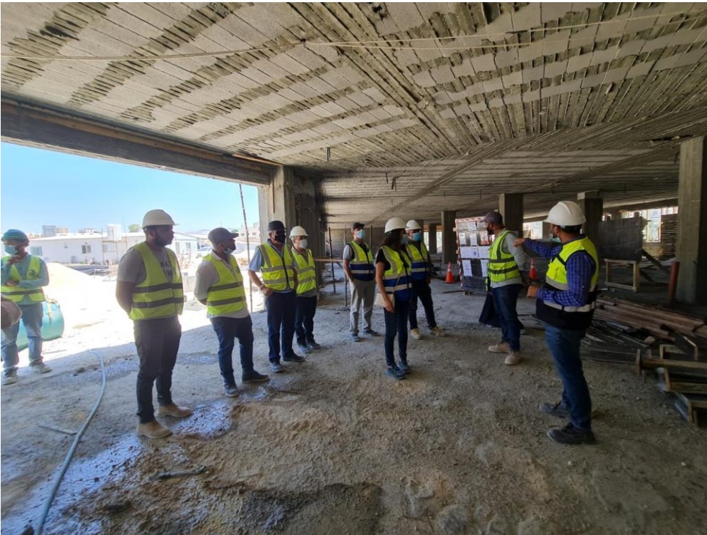
The supervision site engineer gave a brief on the work progress and the current stages and the function of each part
