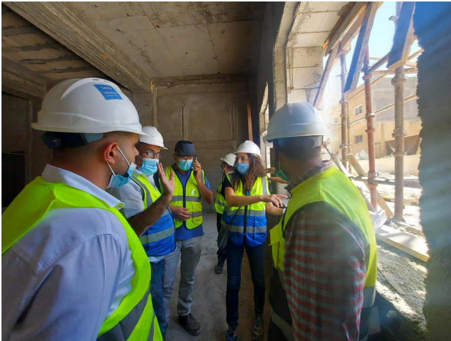
The Consultant discussed with the Contractor window sills details at basement floor, marble/stone
