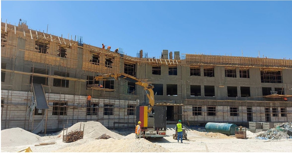
General view of the preparation works for Second floor slab zone "B"
