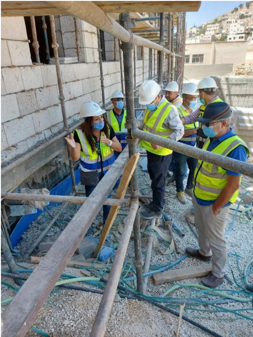
Eng. Representatives observed the executed stone works at the northern, southern, and eastern elevations
