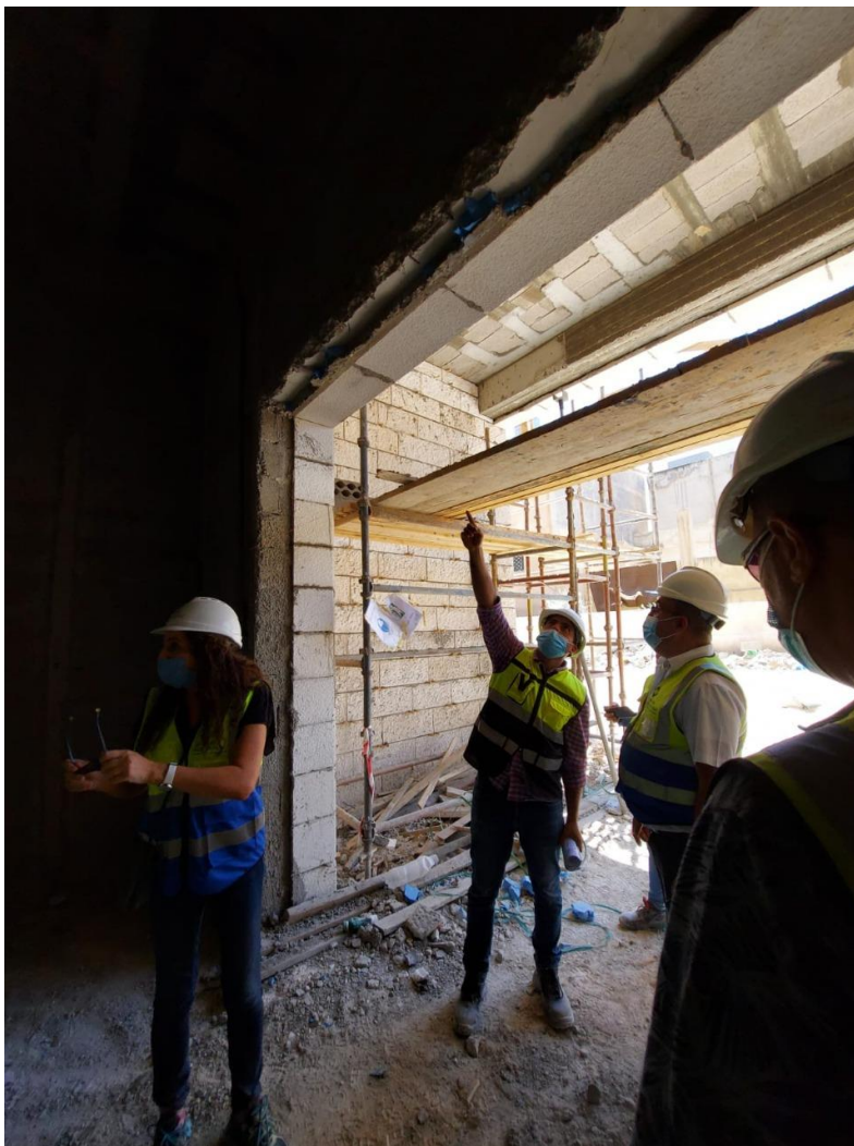
Stone soffit detail and its dimensions over the entry door at entrance
