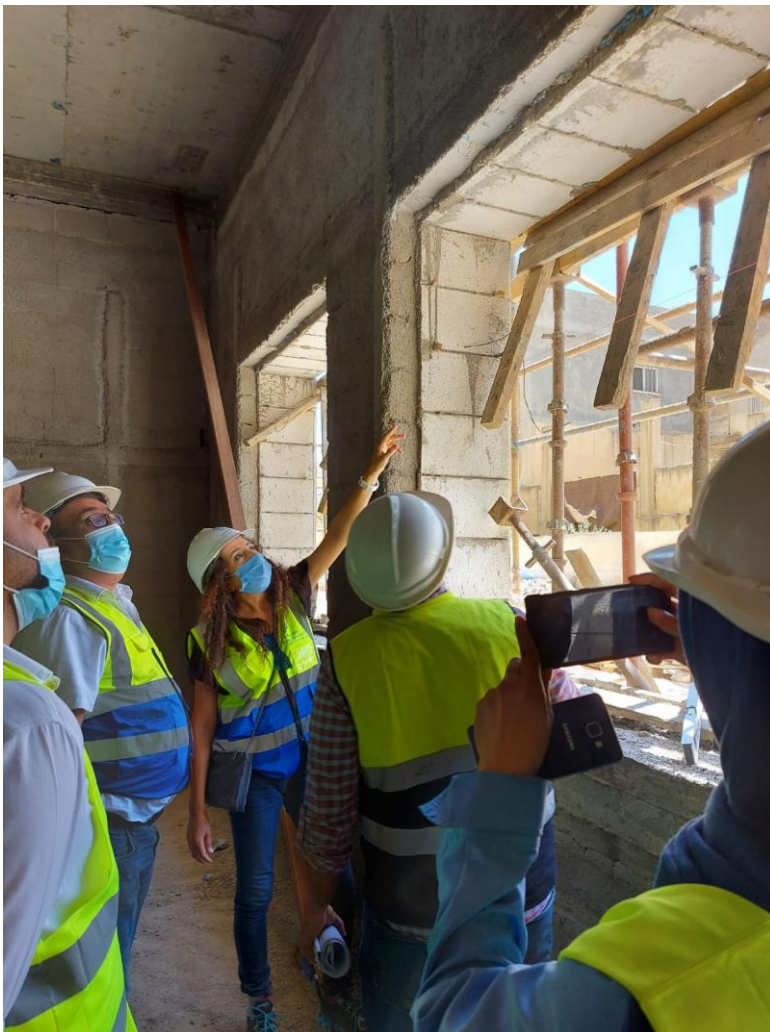
The Consultant discussed with the Contractor the stone soffit detail of one window at basement floor
