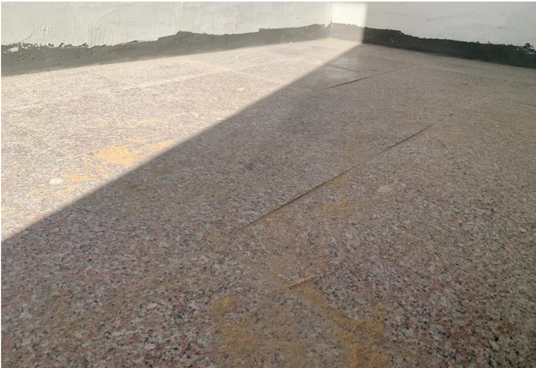
Defected granite tiling
