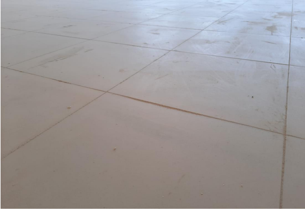
Defected porcelain floor tiles
