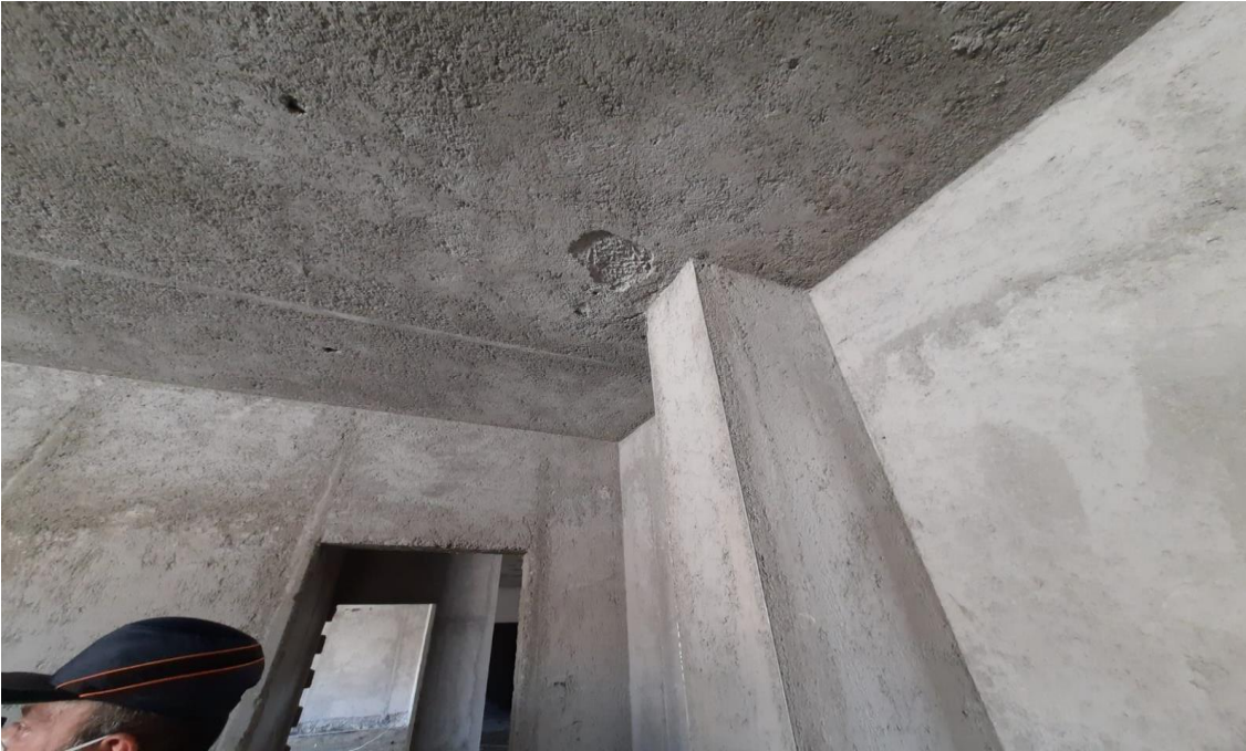
Defects in Plastering
