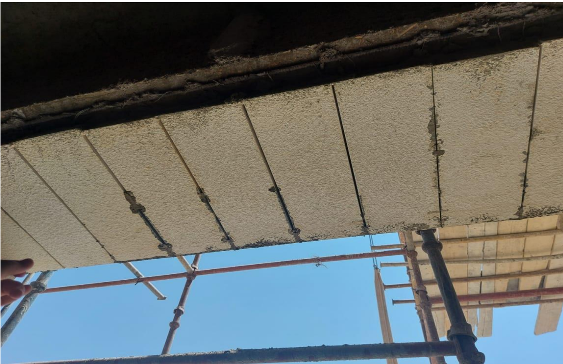
Wide joints in stone soffit
