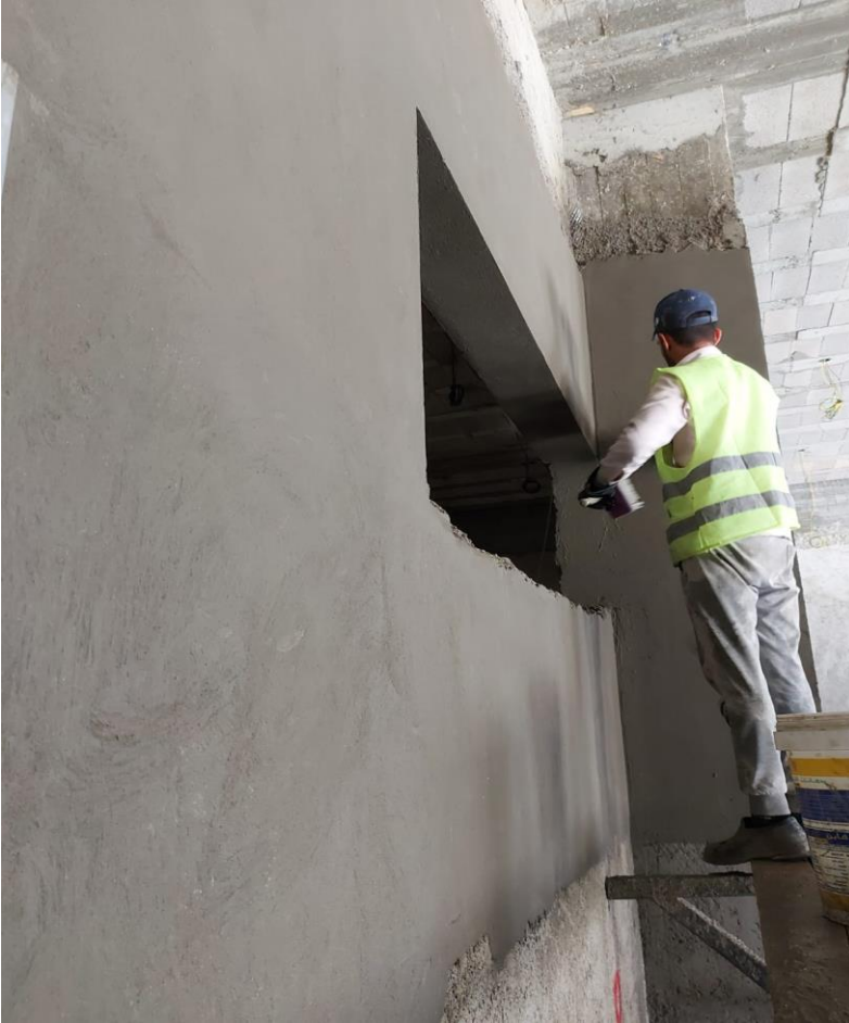
Starting with plastering final finish before completion of rough finish and sill installation
