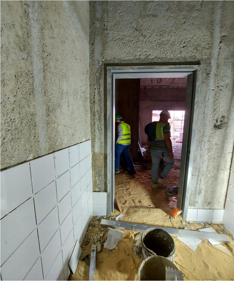
Defects appeared in tiling since no approval was given to the first row
