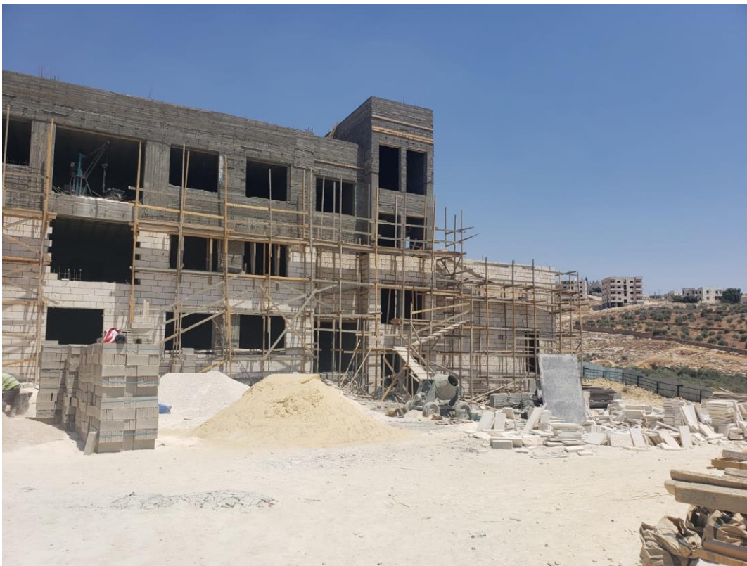
The Contractor is continuing in removing the defected stones to replace them with stones complying with the approved sample. Special zone at the site was identified to sort out the stones and discard the rejected stones. Stone building is still progressing
