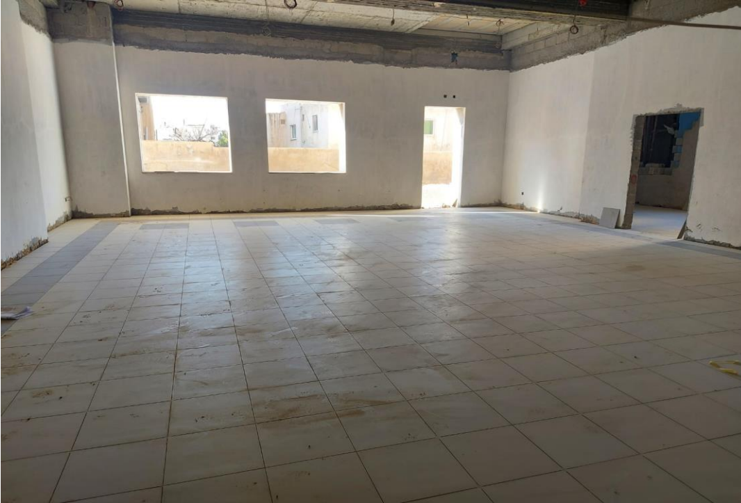
Defected Porcelain floor tiles
