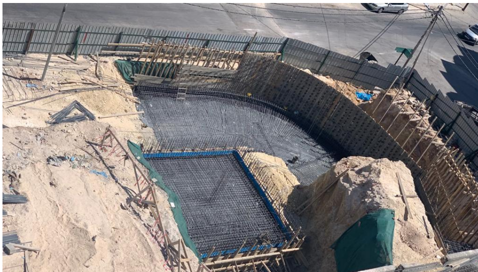
Steel reinforcement for the water tank and the first part of the boundary wall as per the modified plan
