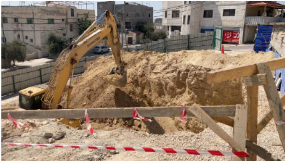
-The Contractor started with the excavation work for external underground water tank
