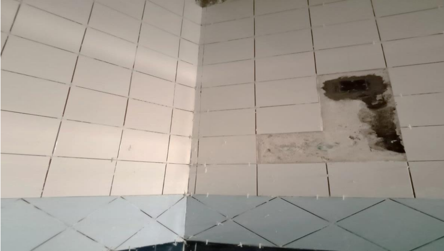
Tiled wall not complying with shop drawings
