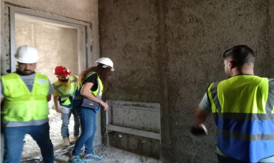
Mechanical cabinet very close to the door frame
