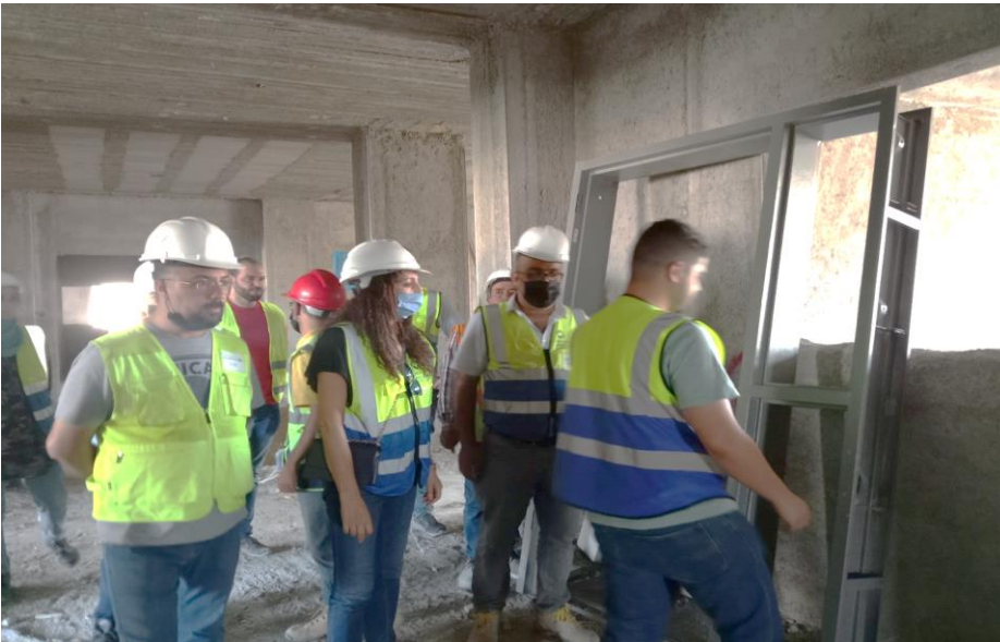
Defected door frames
