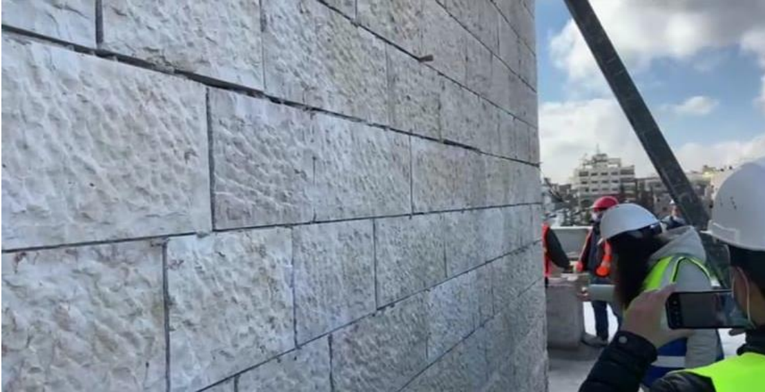
Defected stone works
