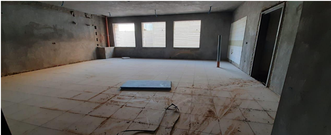
Defected Porcelain floor tiles
