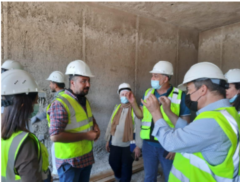
Eng. Hasan/Quality Control Manager explaining how the second layer of plastering shall be executed
