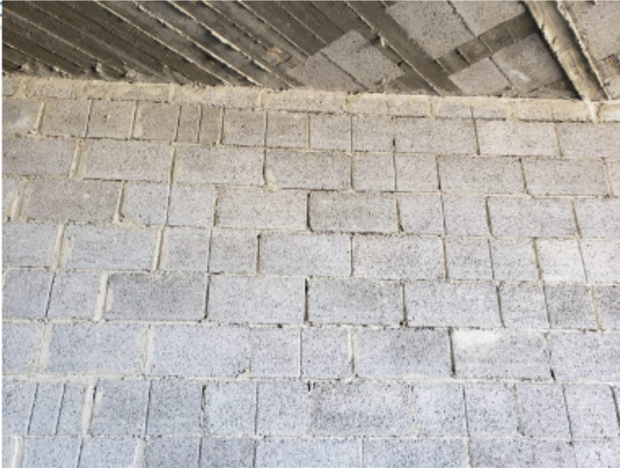
The narrow spaces between block wall and the ceiling is filled with saw cut block
