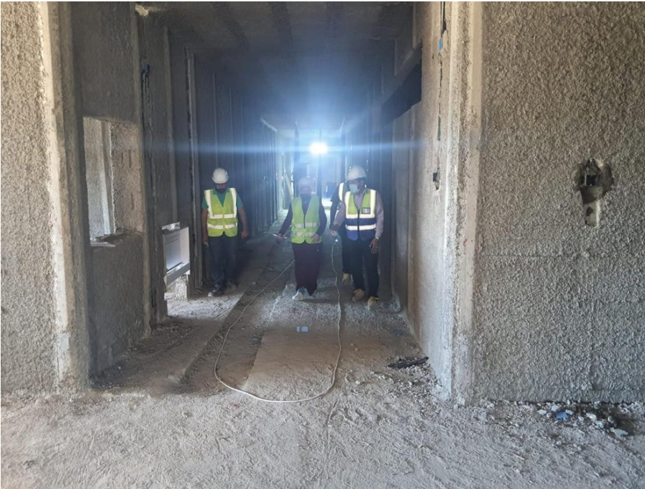
A tour was conducted inside the project in the presence of Eng. Natheer/ Medanat project manager
