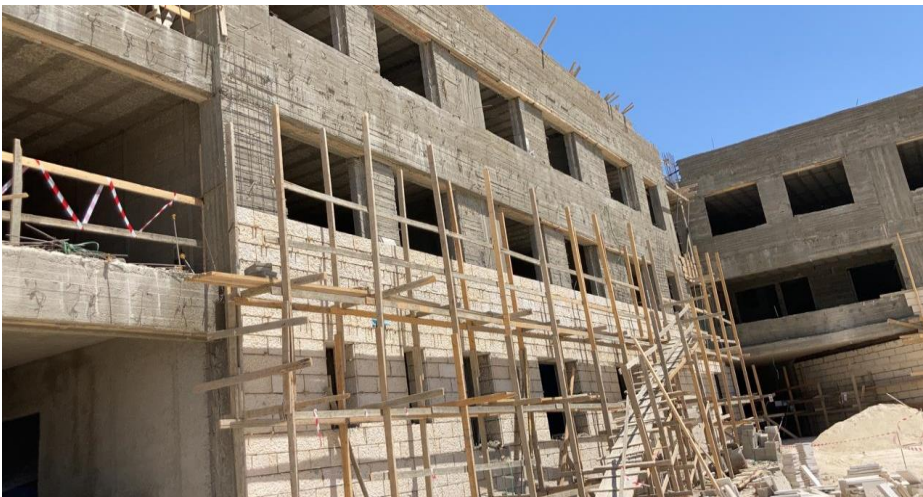
The pattern of stone chiseling should be unified as per the approved sample
