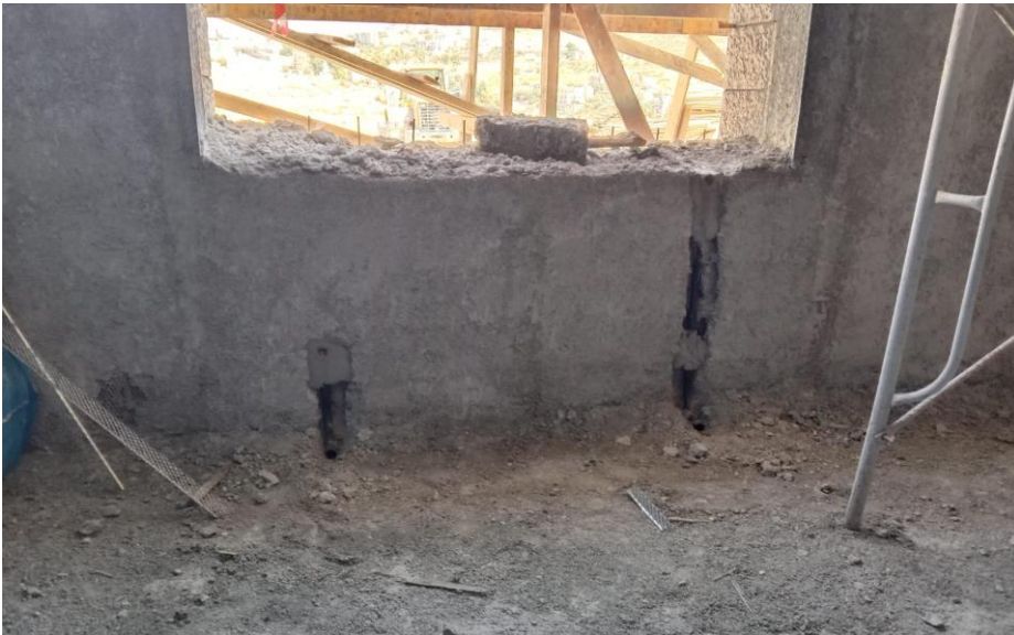
Radiators first fix have been installed top- bottom without approval
