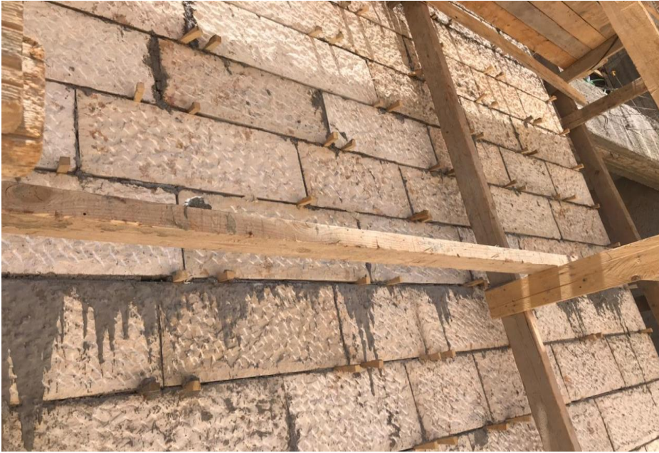
Number of stones are broken, the gaps should be unified and the part of façade is full of cement mortar
