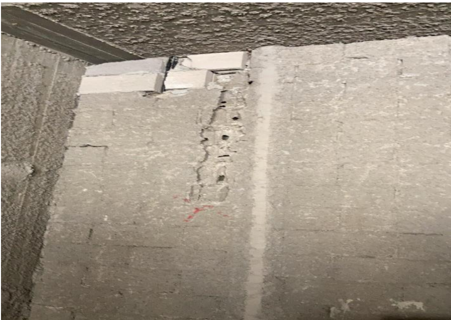
Top layers in block walls are built with defects need to be replaced correctly
