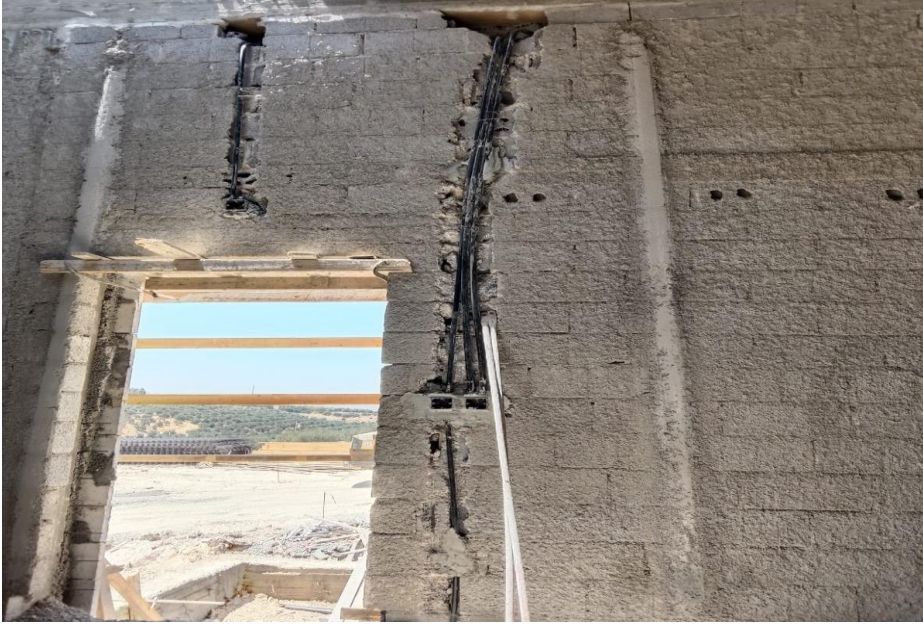
Chipping in block walls are done not saw cut
