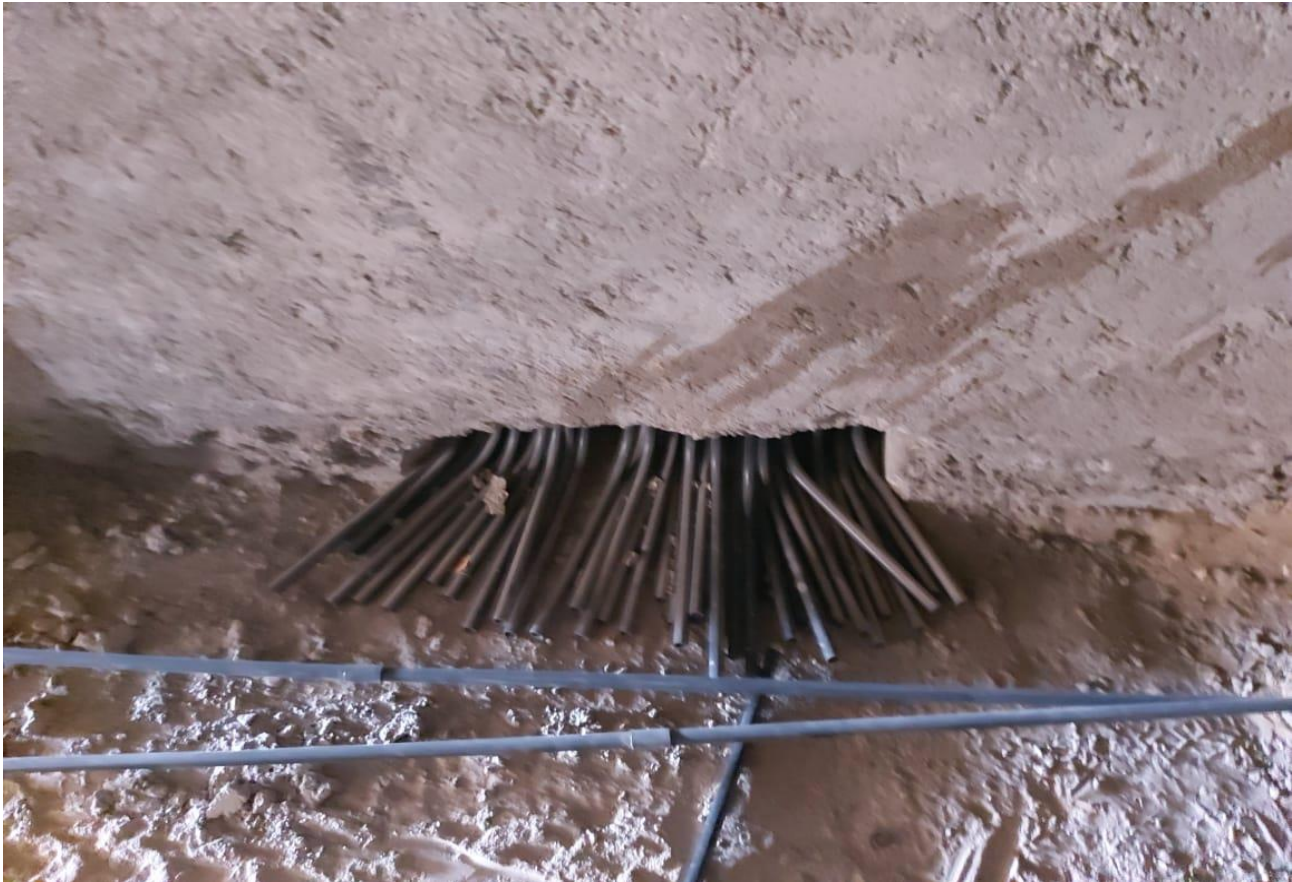
Open electrical pipes
