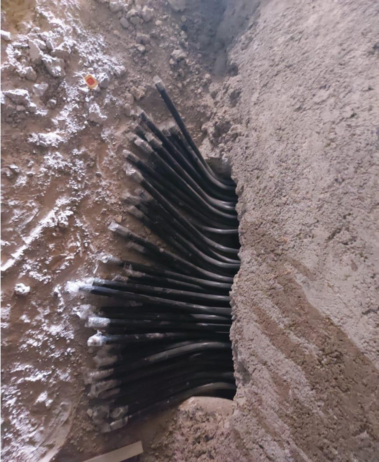
Protected electrical pipes
