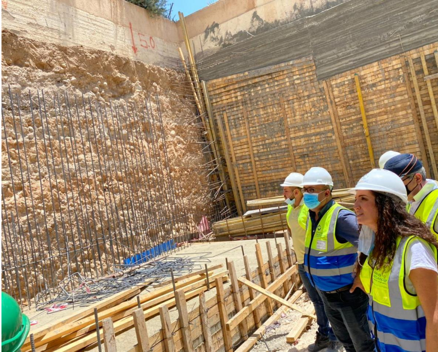
Footing for the new wall adjacent to the existing neighbor's wall is already casted.
