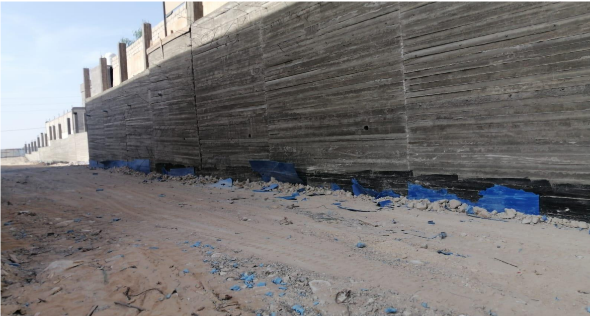
Removal of uncomplied backfilling
