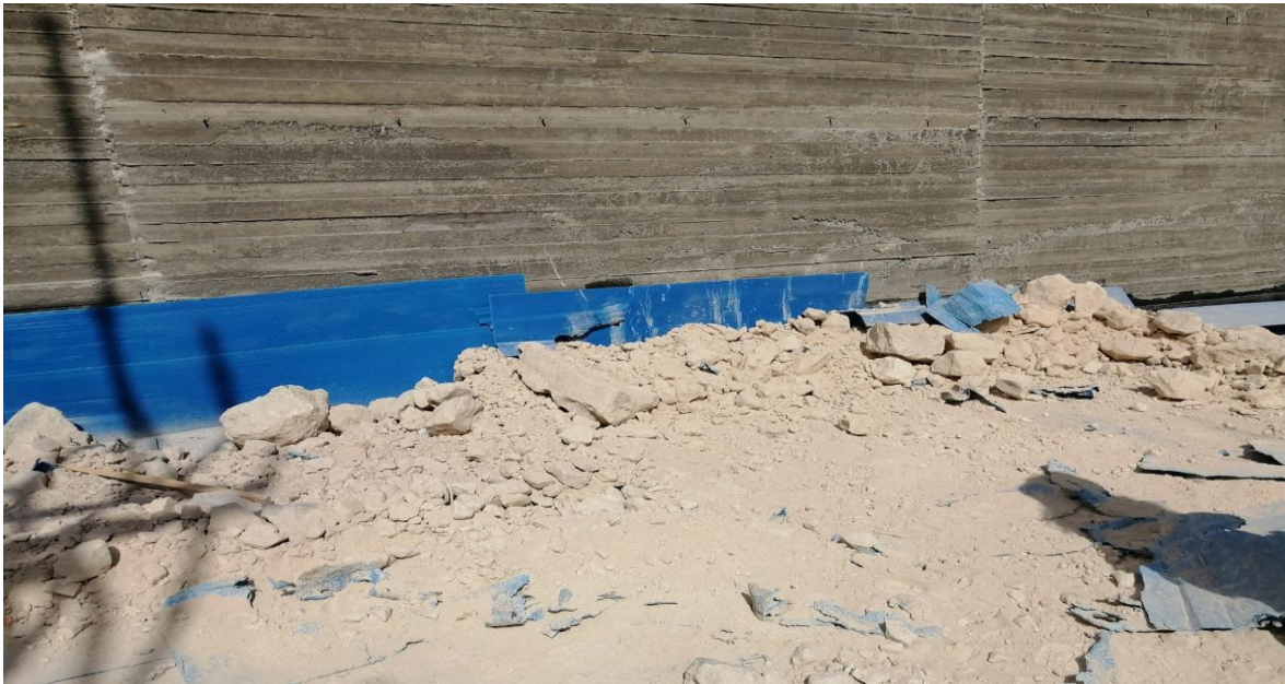
Uncomplimentary backfilling full of boulders
