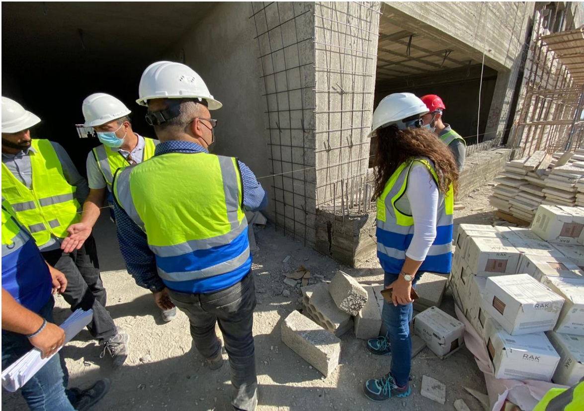
Executing expansion joint wrongly
