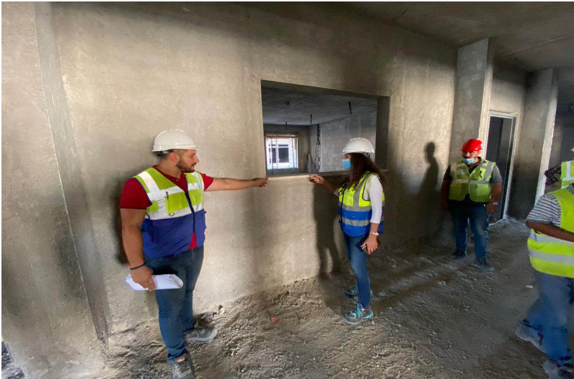
Dimensions of sills are not complying
