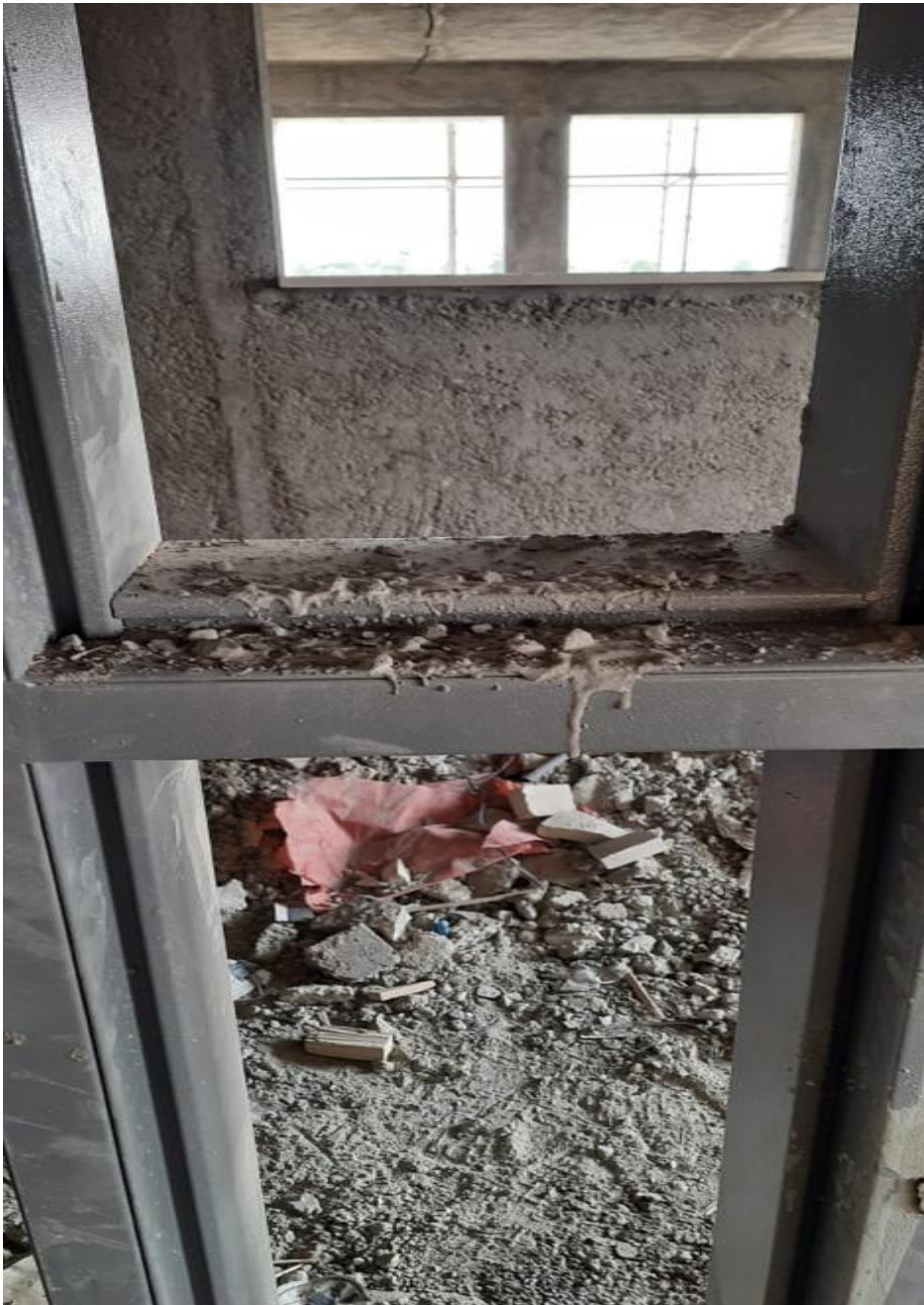
Door frames are not protected
