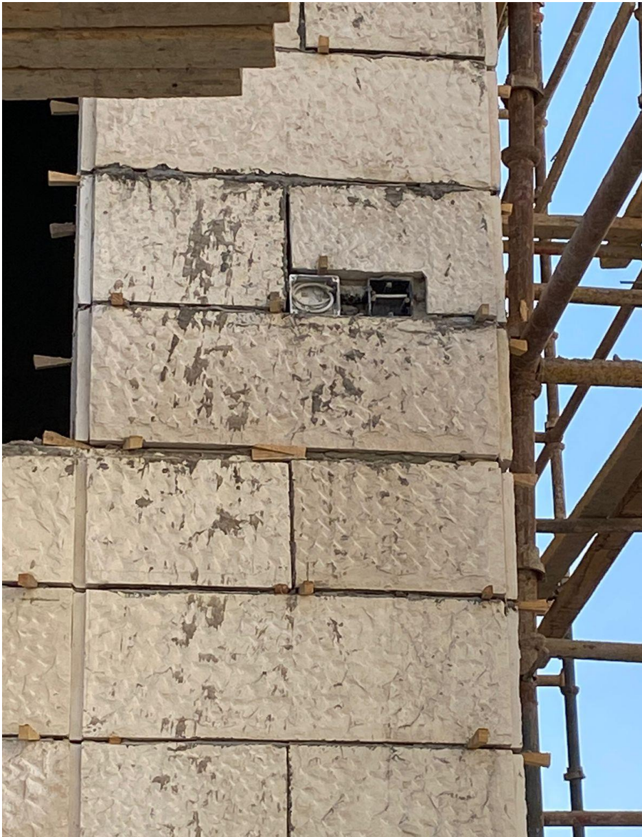
Installing electrical outlets at elevations is wrong
