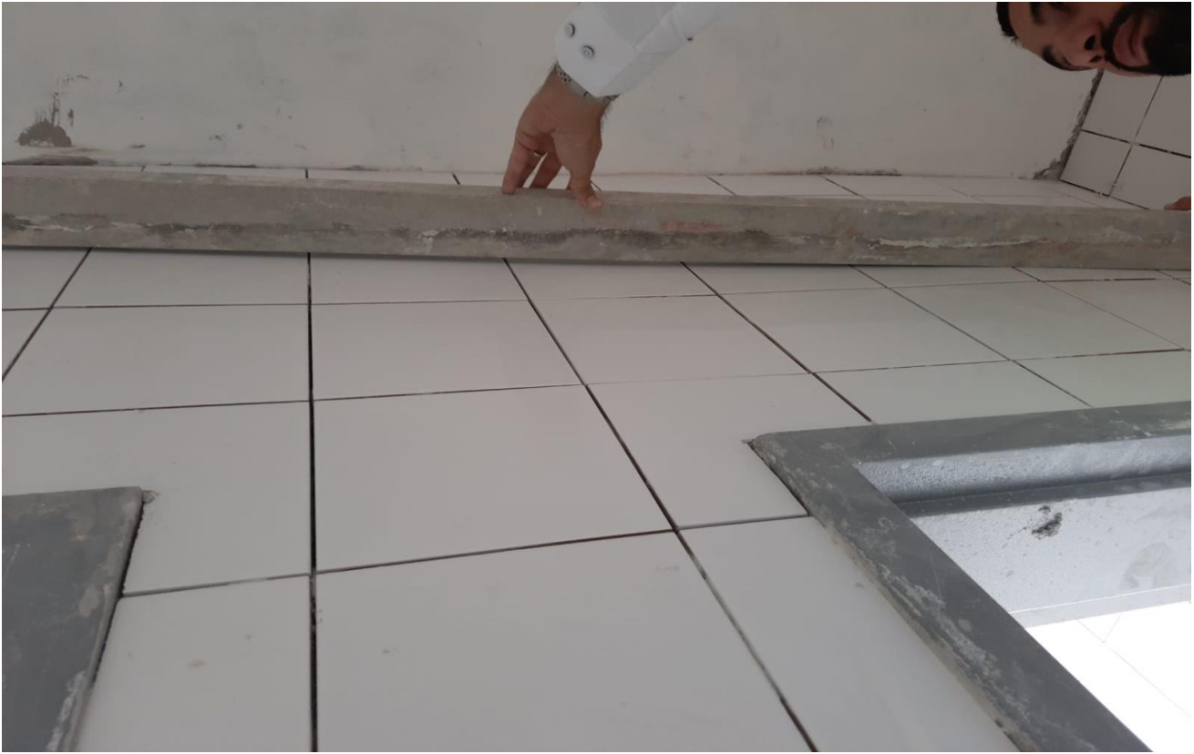
Defected tiling at toilet
