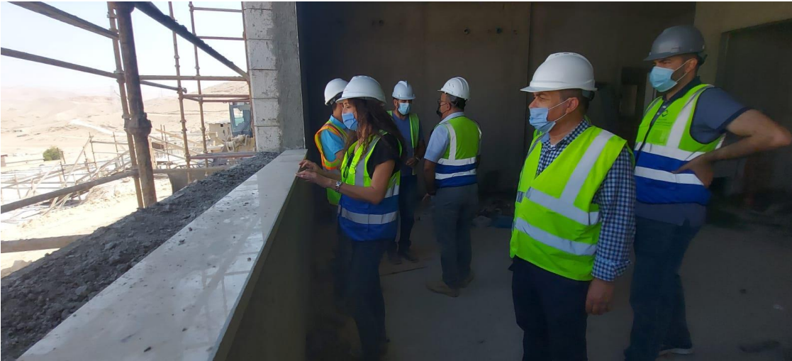
The bottom edge of window sills is toothed and not straight
