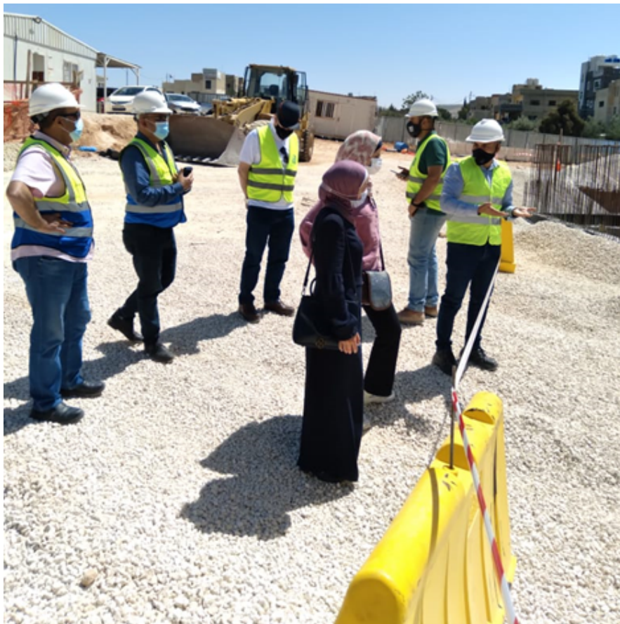
Following up ongoing activities such as: Water tank formwork and ground beams formwork
