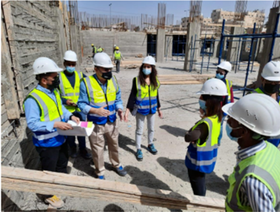
A tour was conducted around the construction site, where Eng. Yousef gave a brief about ongoing works
