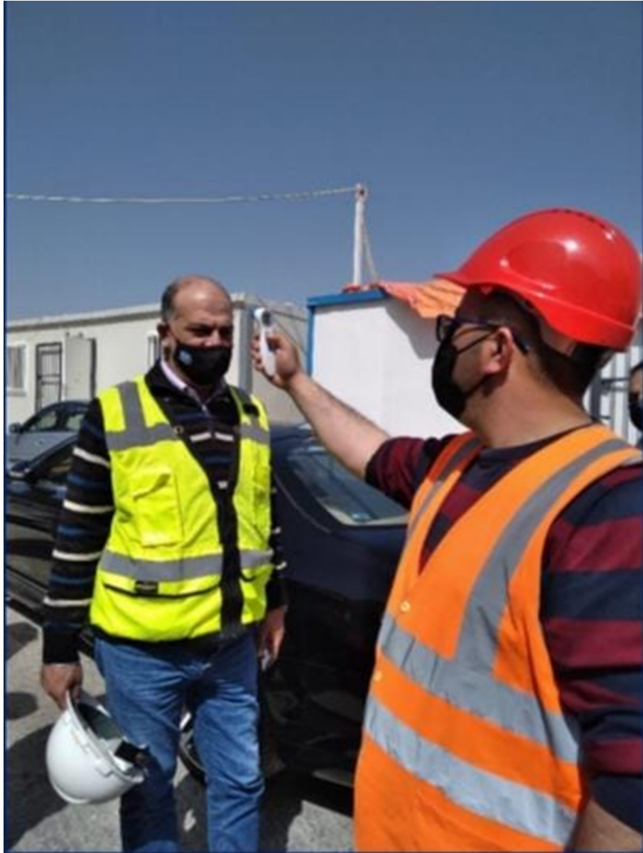
Temperature check at the entrance of the site, complying with Covid-19 Protocol
