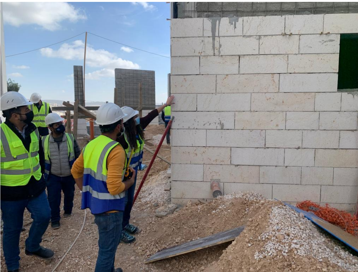
The executed stones for facades have been inspected in general and remarks have been given to the Contractor to rectify where necessary
