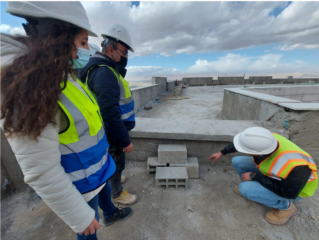
The supervision team observed that the Contractor progressed in the work of expansion joints at the roof between zones A and B
