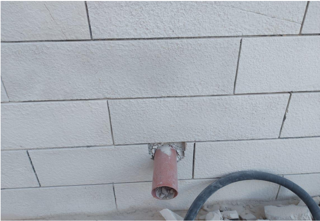
Defected stone around the pipe
