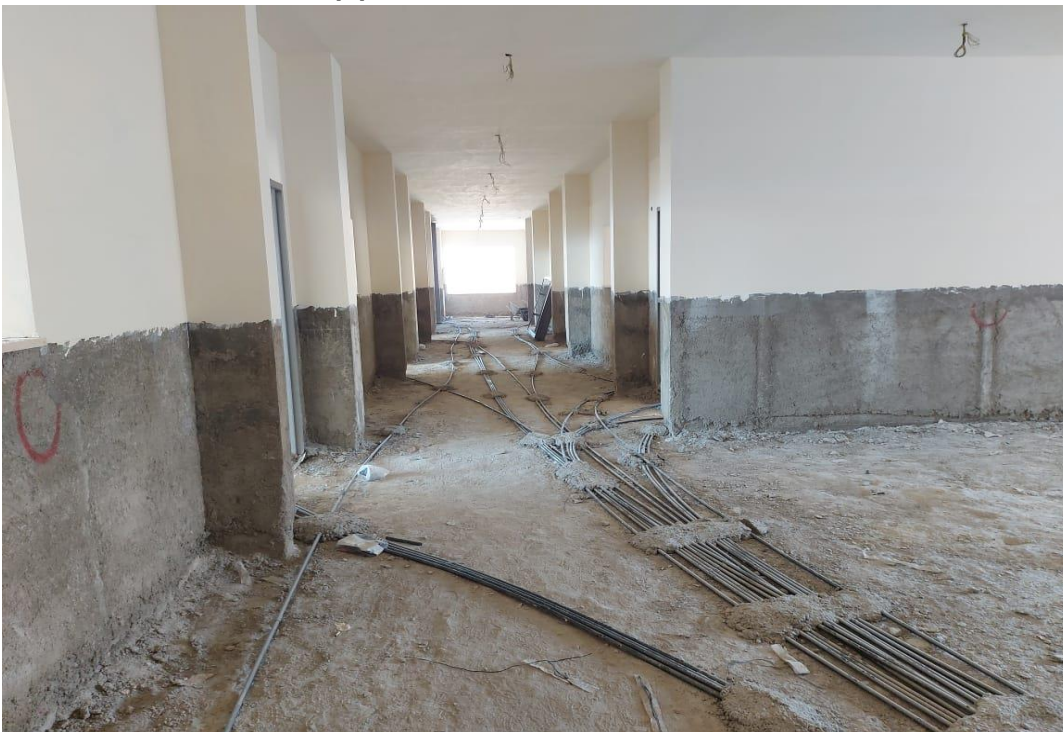
Un-protected electrical pipes
