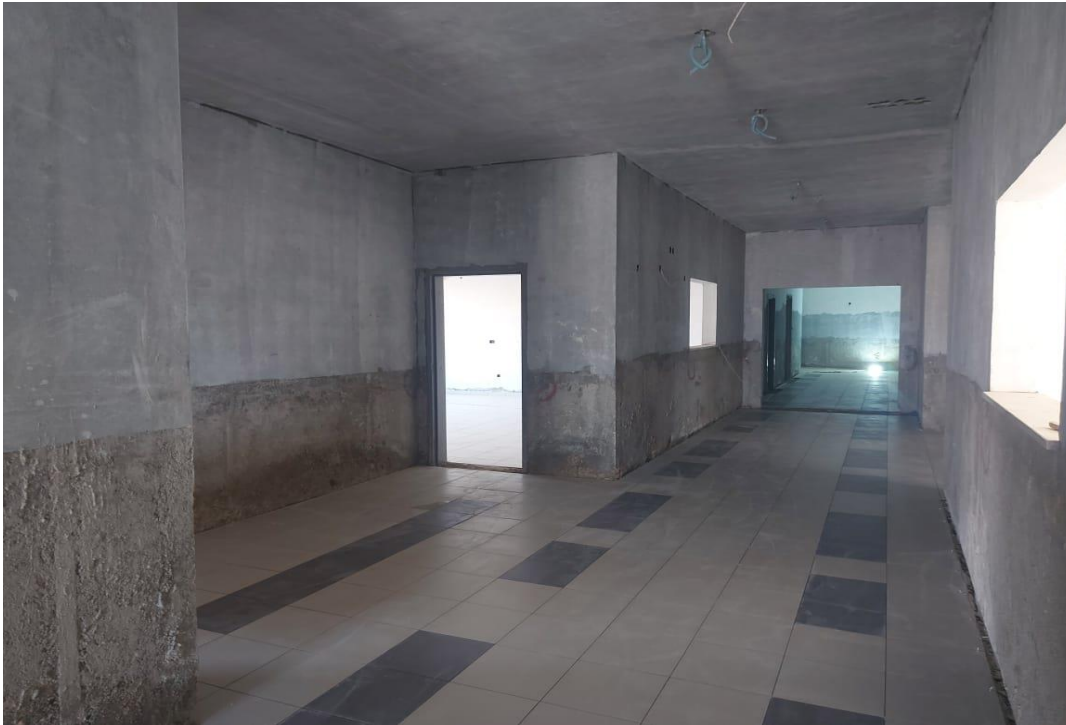
Defected floor tiles
