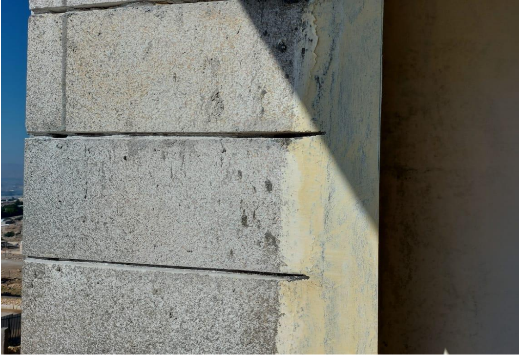
Defected plastering work
