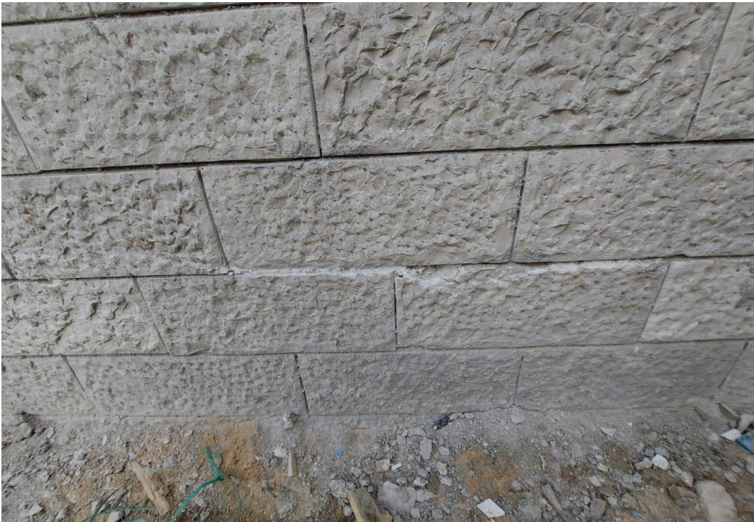
Defected stone work
