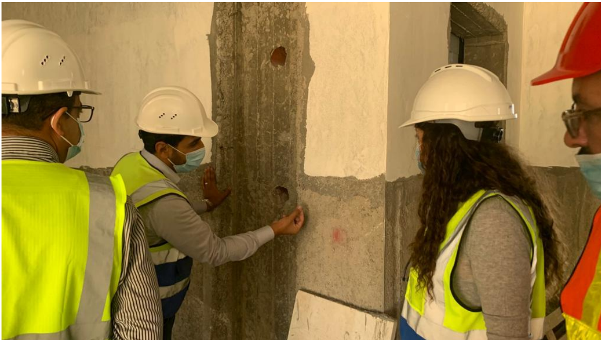
The electrical engineers from the supervision and the Contractor discussed the location and the method of installation for the elevator control panel
