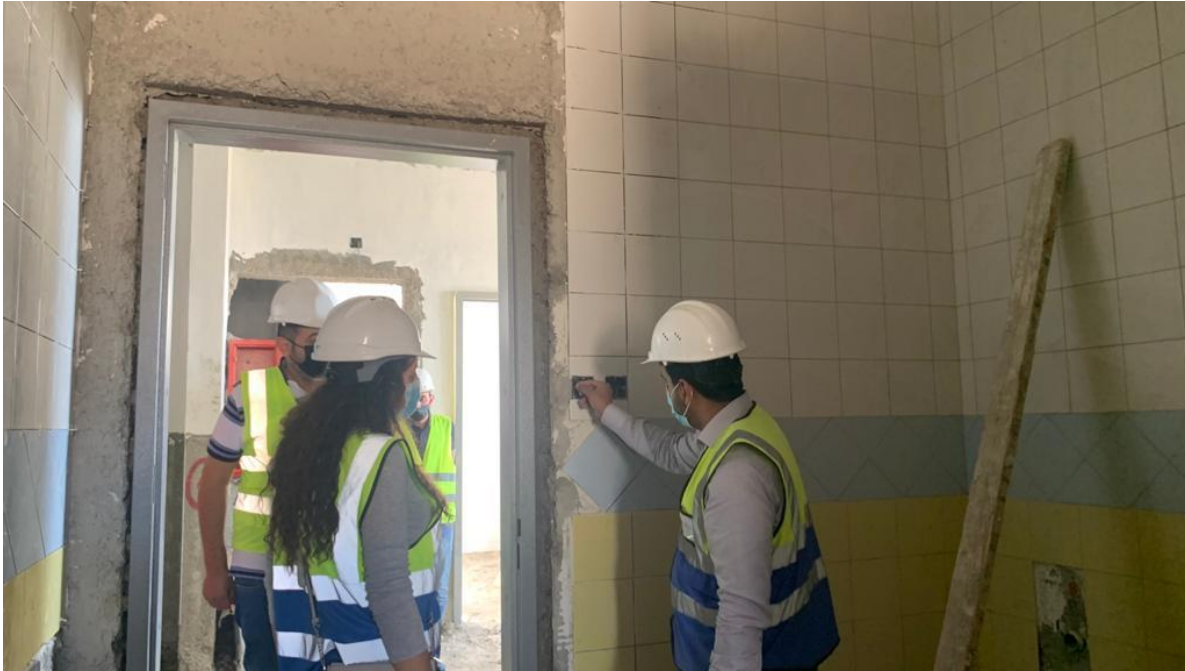
The location of electrical sockets was discussed in relation to the wall tiles
