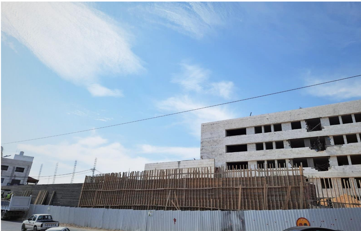
After removing the electrical poles (previous obstacle) on 03/10/2021, the external works continued as shown
