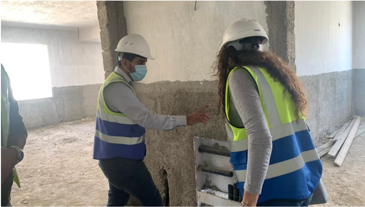
The installation of mechanical cabinets was checked also at the corridors
