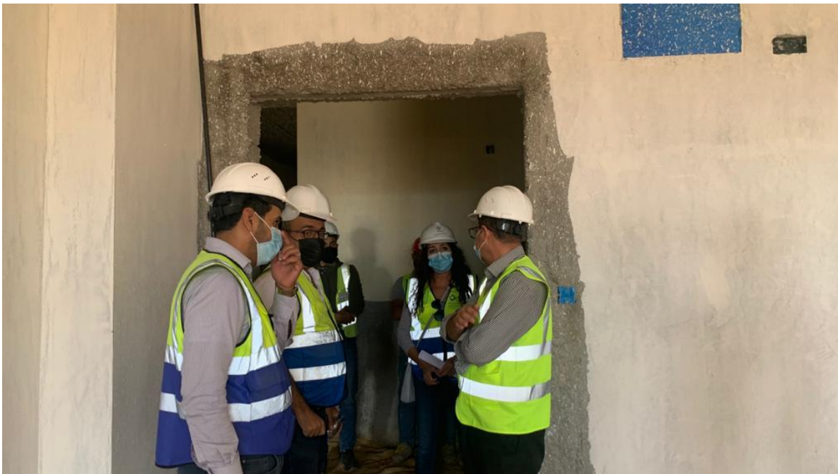
The visiting team observed the delay in delivering the remaining steel door frames
