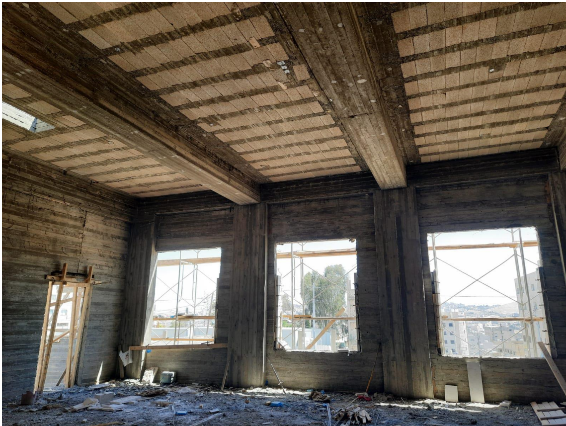
It was observed that the Contractor is striking the formwork of the multipurpose hall (theater) roof
