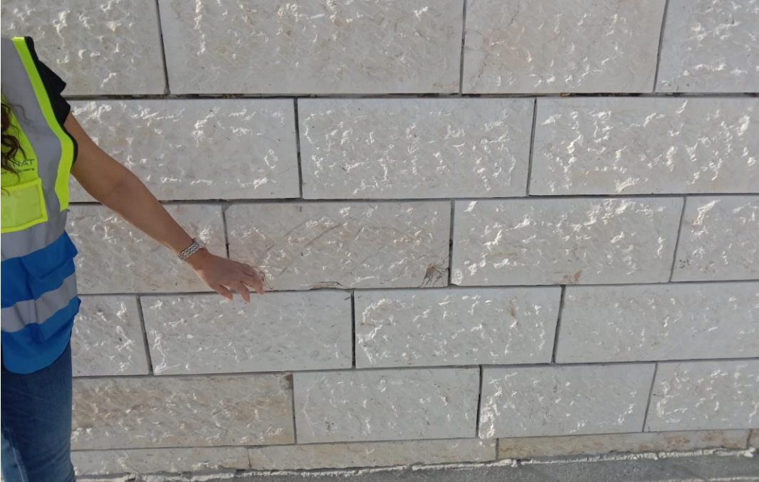
Defected built stones
