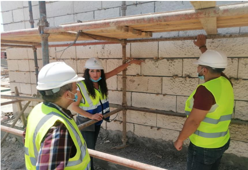
The texture of number of stones do not match with the approved sample
