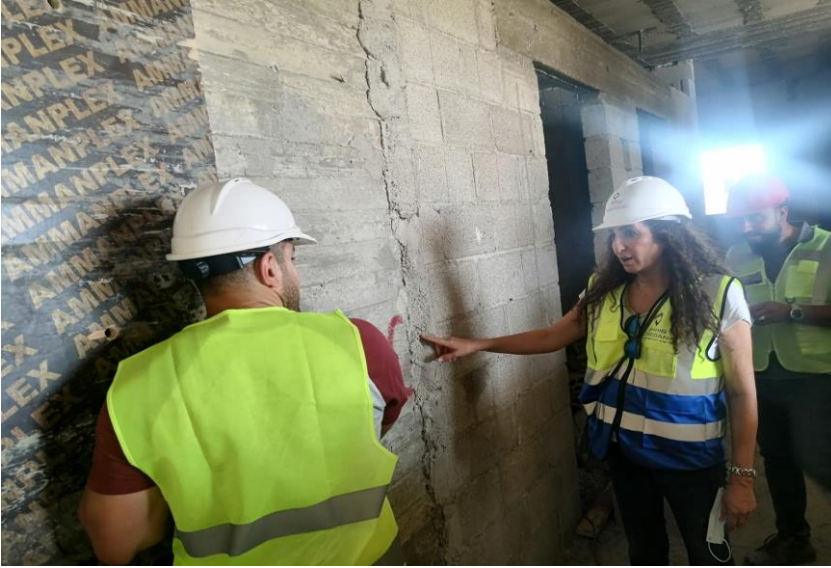
The Blockwork is not in line with the Concrete Wall
