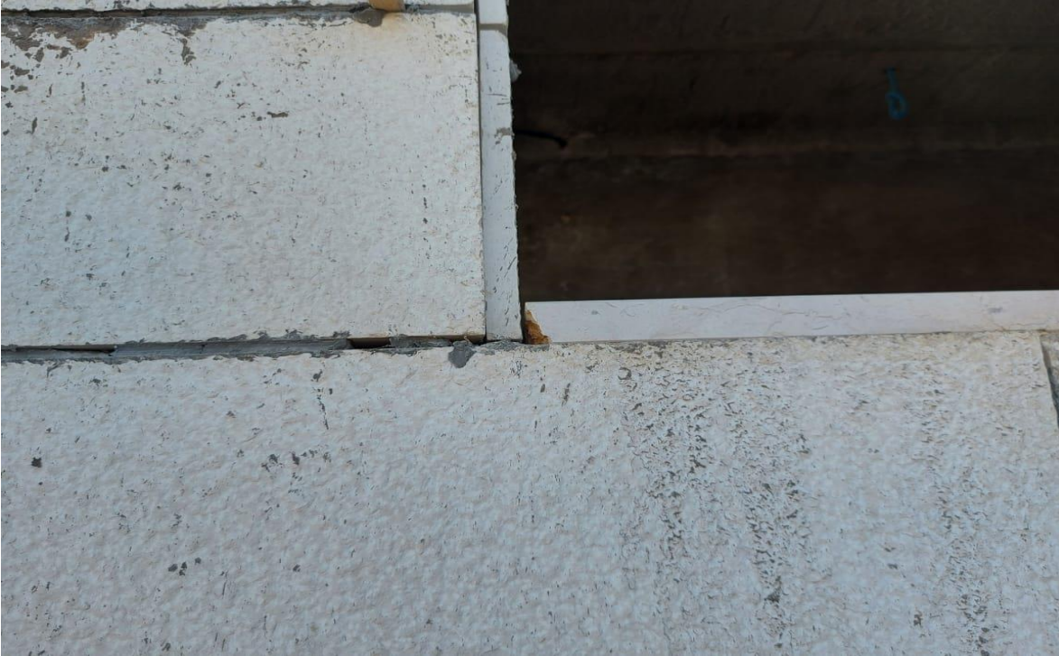
Broken window sills
